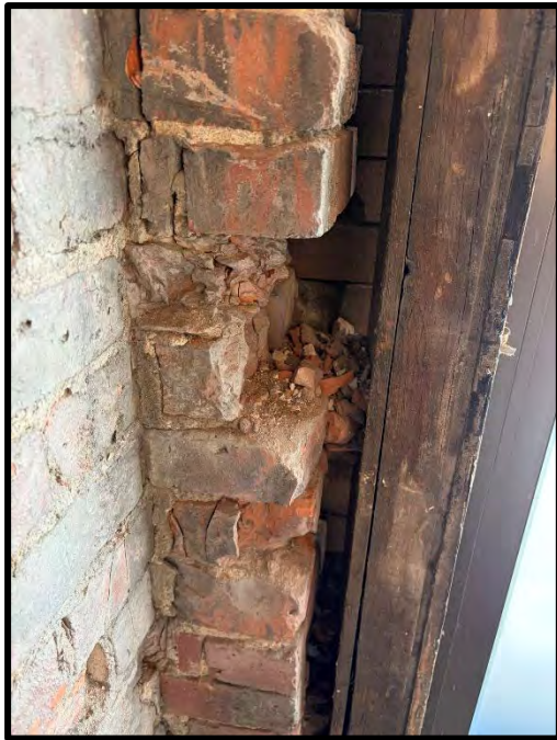
Figure 2e (left) Fifth floor missing brick at window jamb
