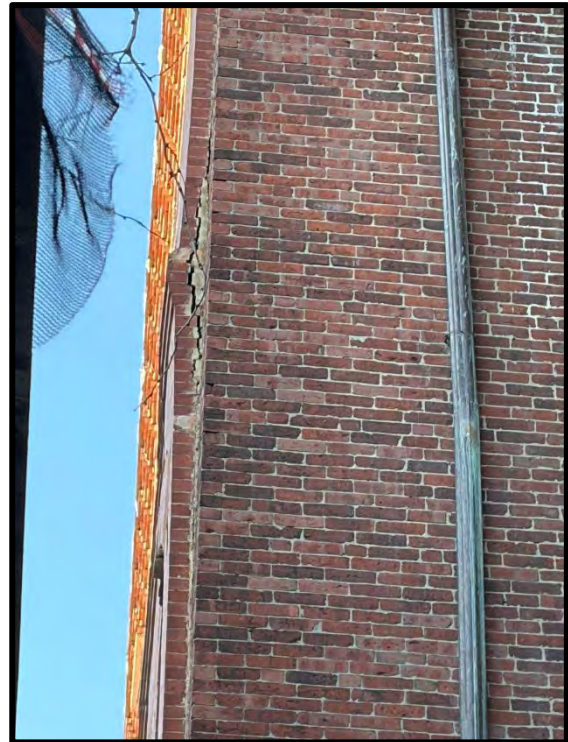
Figure 1d (right) East façade (facing 401 Shawmut Avenue) showing the fourth floor water table cracked and pulling away from the building
