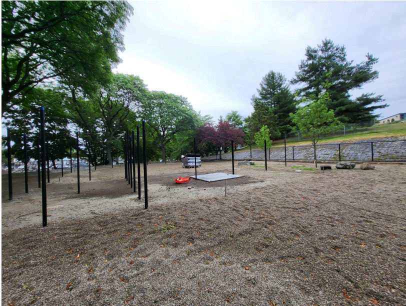
The new dog park surfacing and fencing is being installed. Trees have been planted.
