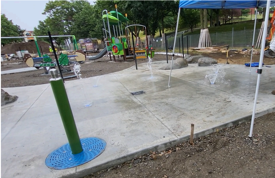
The new sprayground is being tested.
