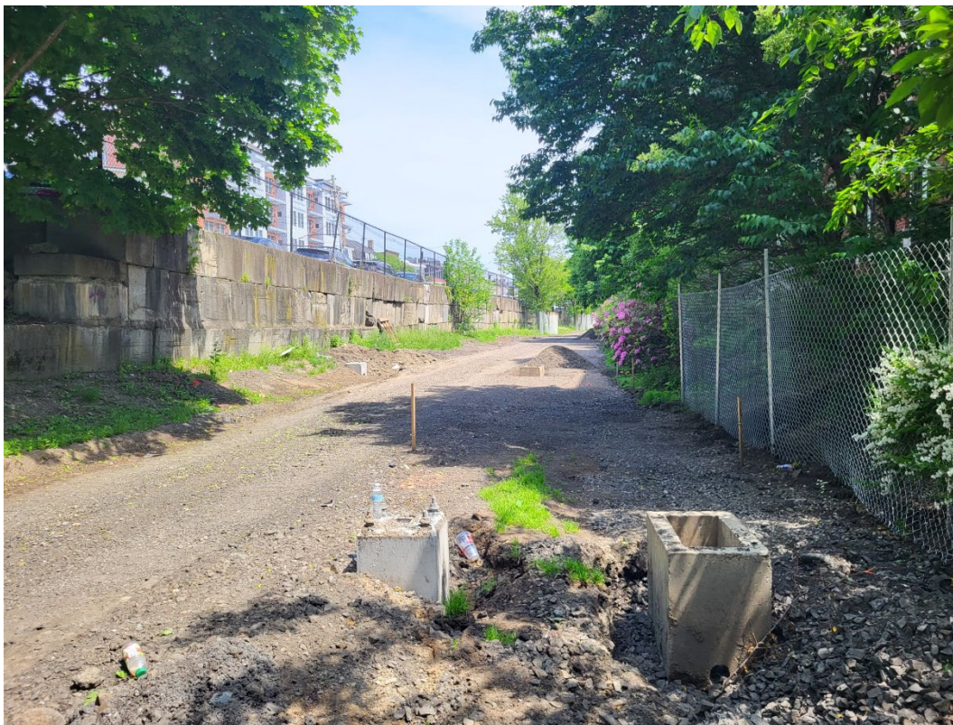
Light pole footings and electrical hand holes have been installed along the path
