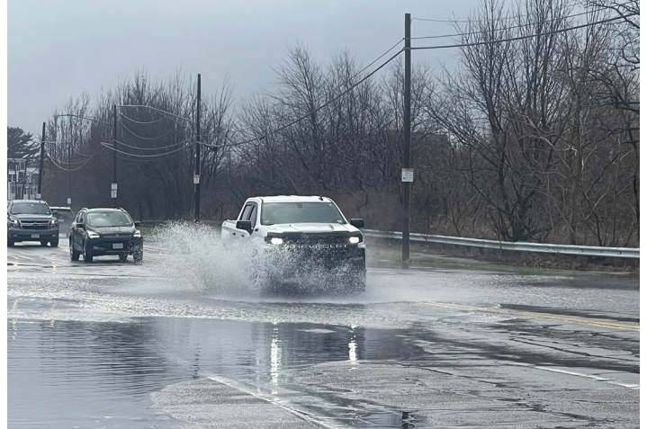
Flooding overtopping Bennington Street, looking southbound towards East Boston.
