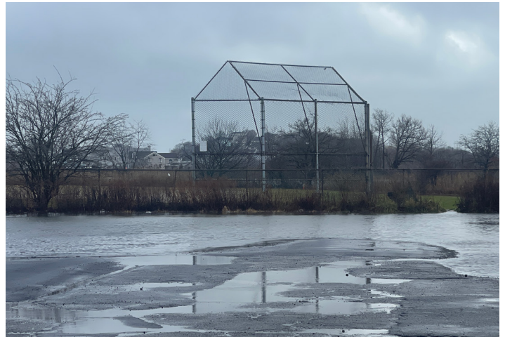
Flooding in the VFW Property parking lot, facing Fredericks Park in Revere.
