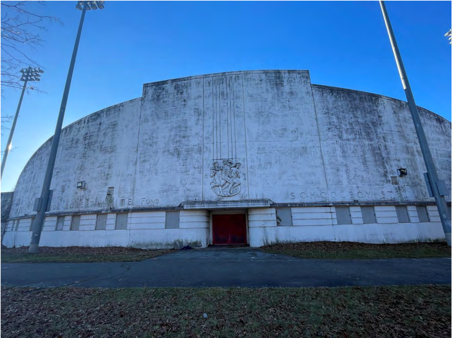
Photo 1. Image of existing stadium infrastructure on the eastern side of White Stadium.
