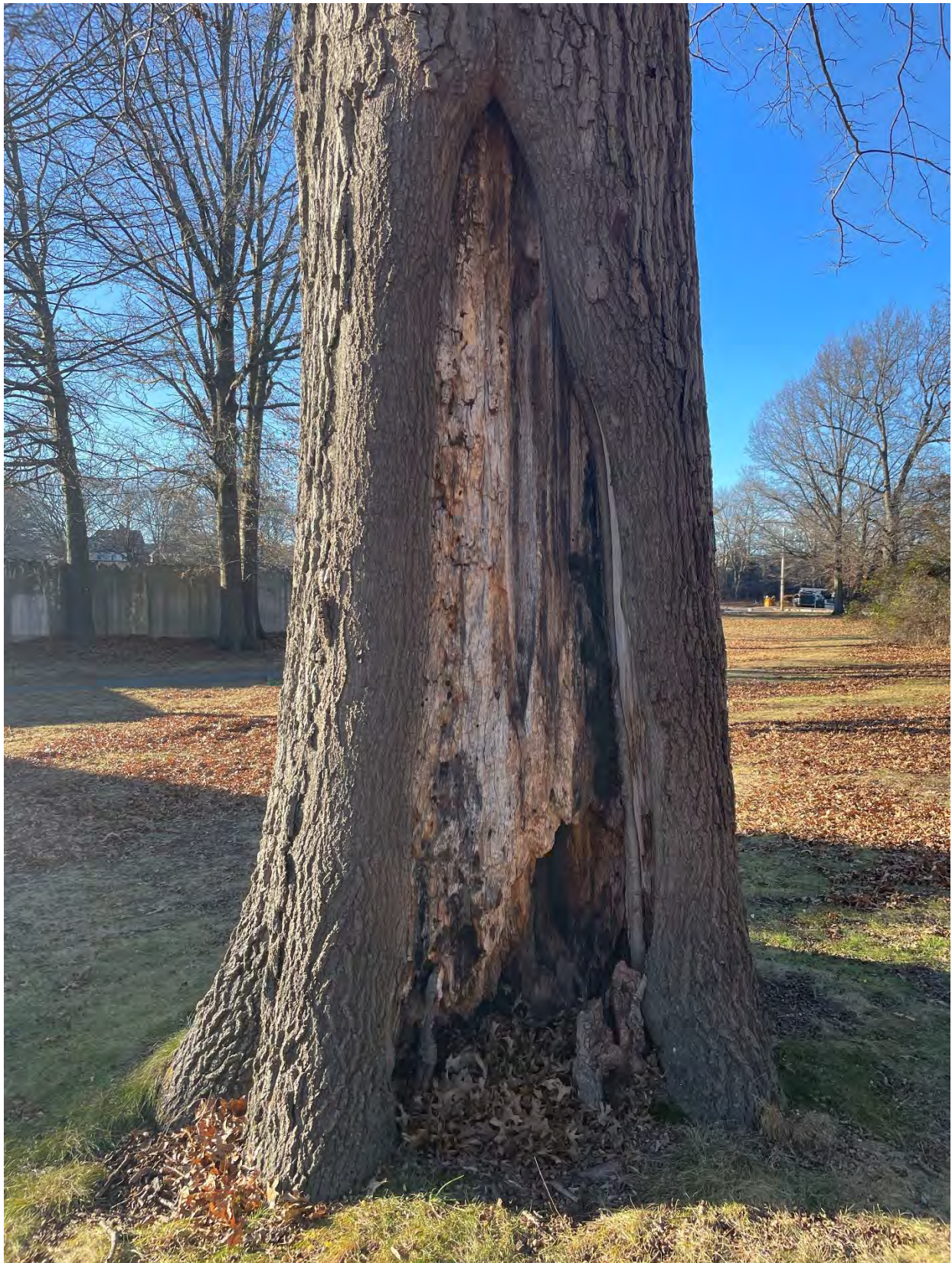
Photo 5. Image of Tree 16. This tree was the largest tree observed in the site area. It was determined that this tree has a low suitability for preservation because of extensive stem decay.
