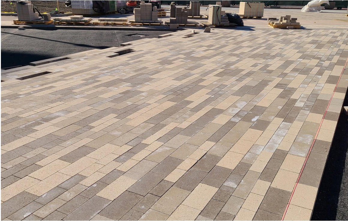
The pavers are being installed in the main plaza, with our new pavers! The colors look much better, and complement the tones of Trinity Church, Old South Church, and the Library building.
