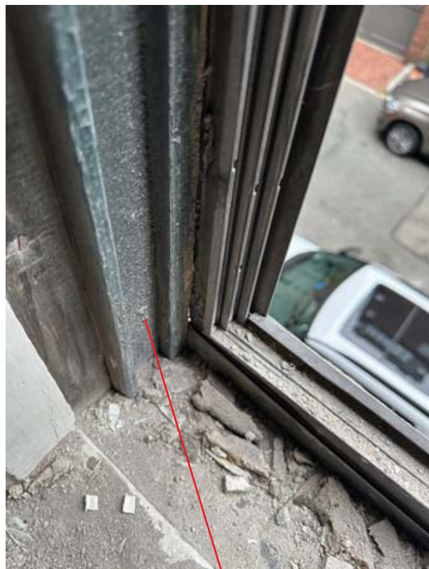
Degradation of wood jamb
