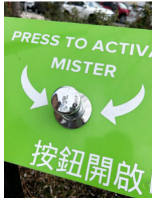
Example of a metered water valve. This type of valve is set to dispense water for a defined amount of time, meaning there is no risk of water being left on.
