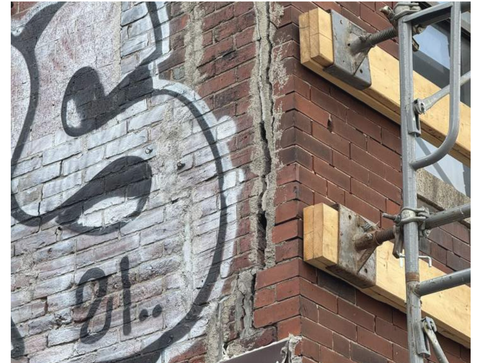
SEPARATION OF MASONRY WALLS
