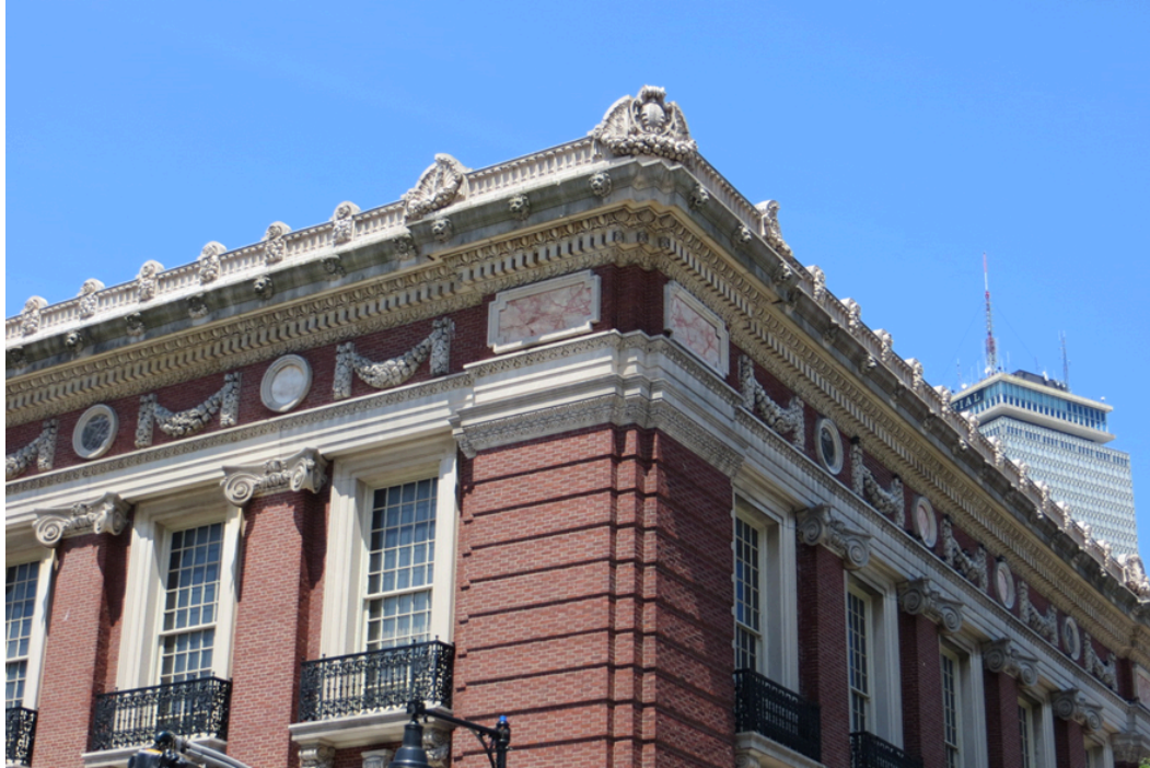
Figure 5. Entablature and cheneau at the corner of south and west façades (looking northeast). July 2016.
