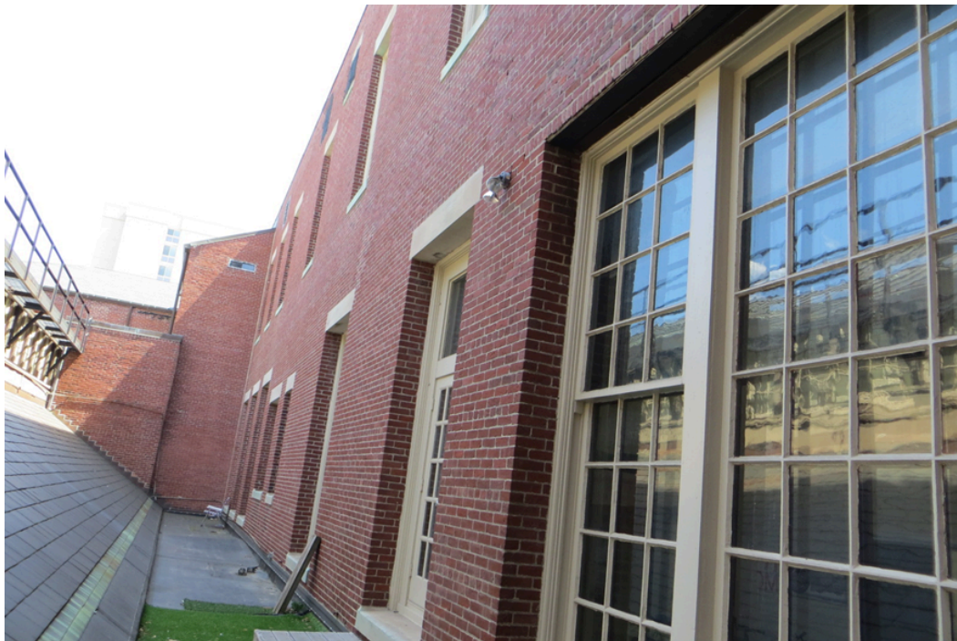
Figure 12. East elevation second story and attic level windows (from first story roof, looking south). July 2016.
