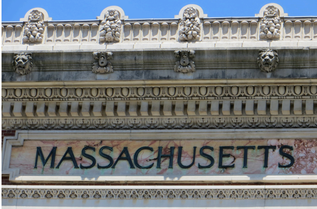
Figure 7. Detail of cheneau and cornice on the west façade (looking east). July 2016.
