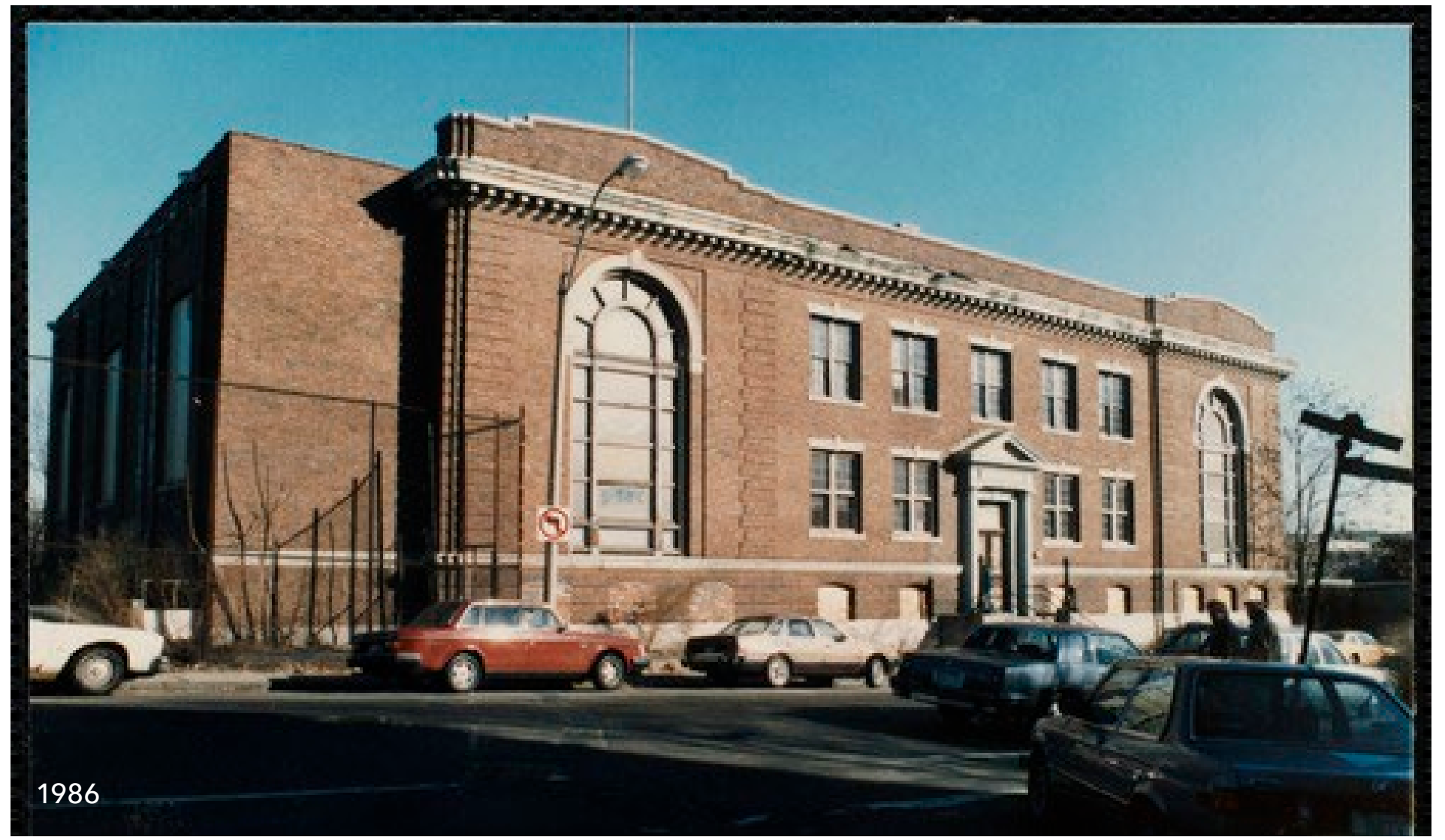
PRIMARY FACADE 1913 PRESERVE HISTORIC SOUTHWEST FACADE IN-KIND, MATCH HISTORIC DETAILS AND FINISHES
