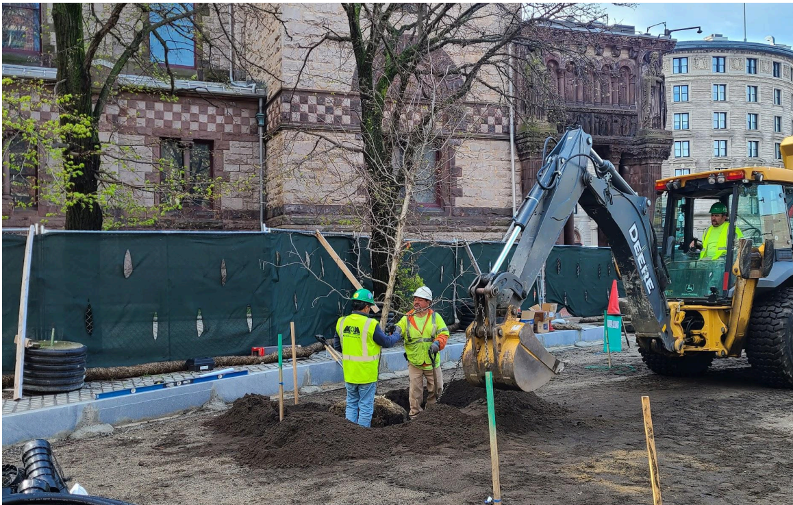
The planting area adjacent to Trinity Church will be paved with a porous gravel pavement, so these trees get installed first. This swamp white oak is part of a stand of 7 trees.
