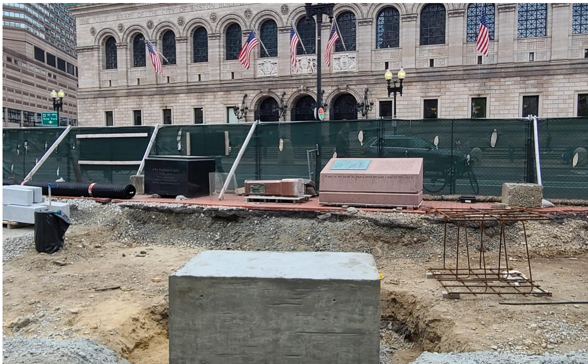
The Kahlil Gibran memorial will now be oriented so that the viewer sees the Library building beyond, reflecting the important relationship between the poet and this beloved institution. In this photo, you can also see the over-excavation surrounding the memorial base, which is where our next planter will be installed.
