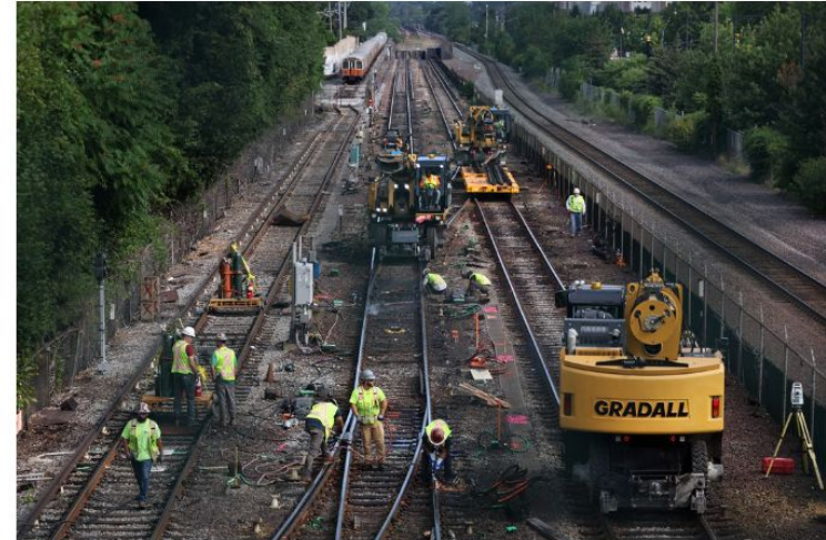
Crews worked on the tracks at the Wellington MBTA station in Medford on Saturday. CRAIG F. WALKER/GLOBE STAFF
