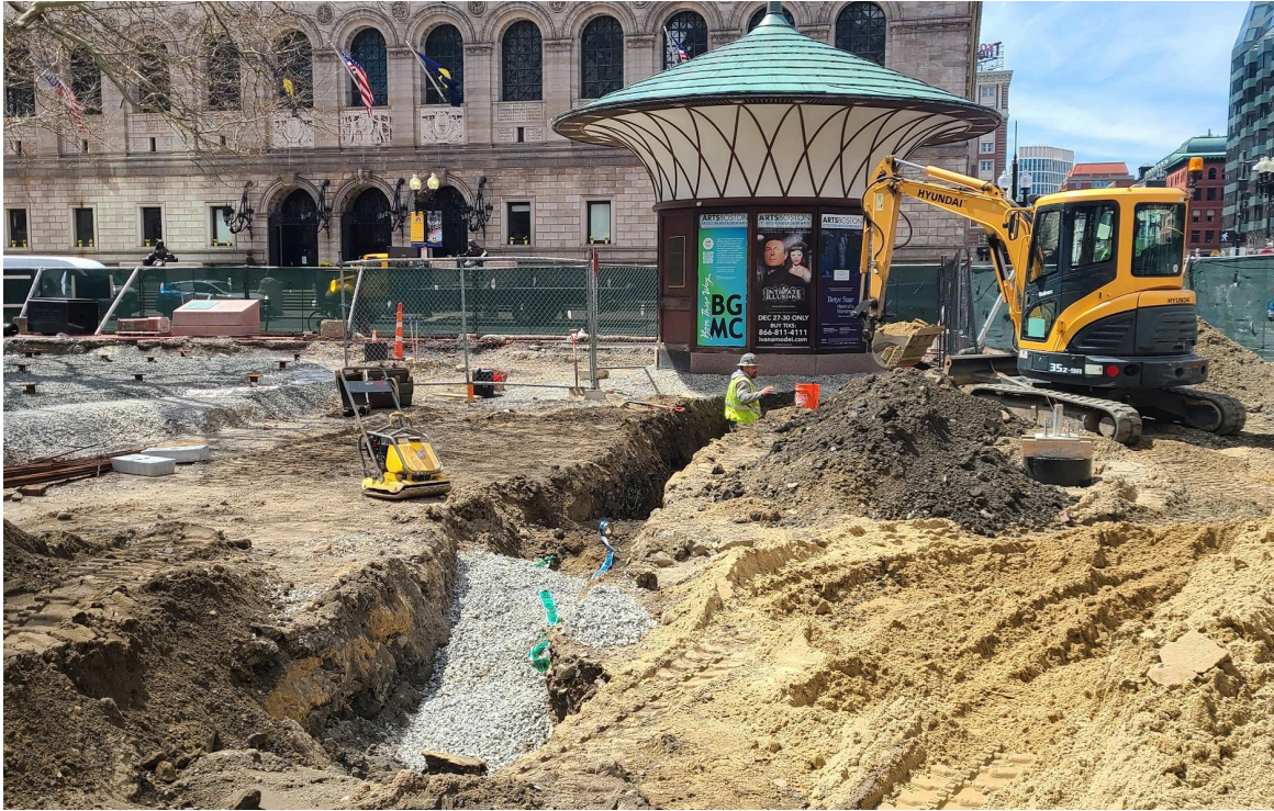
A four-foot deep trench is dug to receive the new water line for the kiosk.
