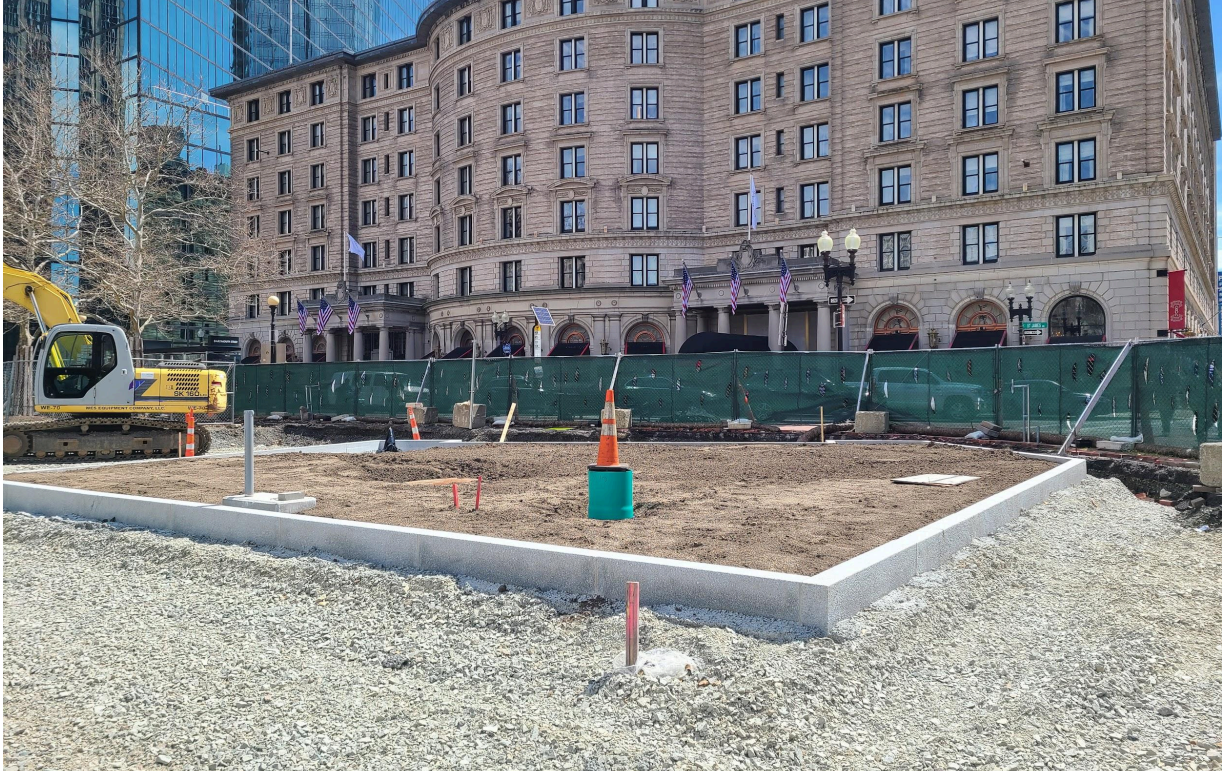
Curbs and soil are complete for the new planter at the corner of Dartmouth Street and St. James.
