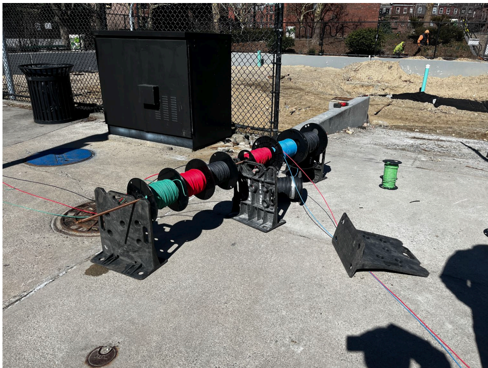
Our electrical team is installing new wiring and testing the existing system to make sure it meets code.
