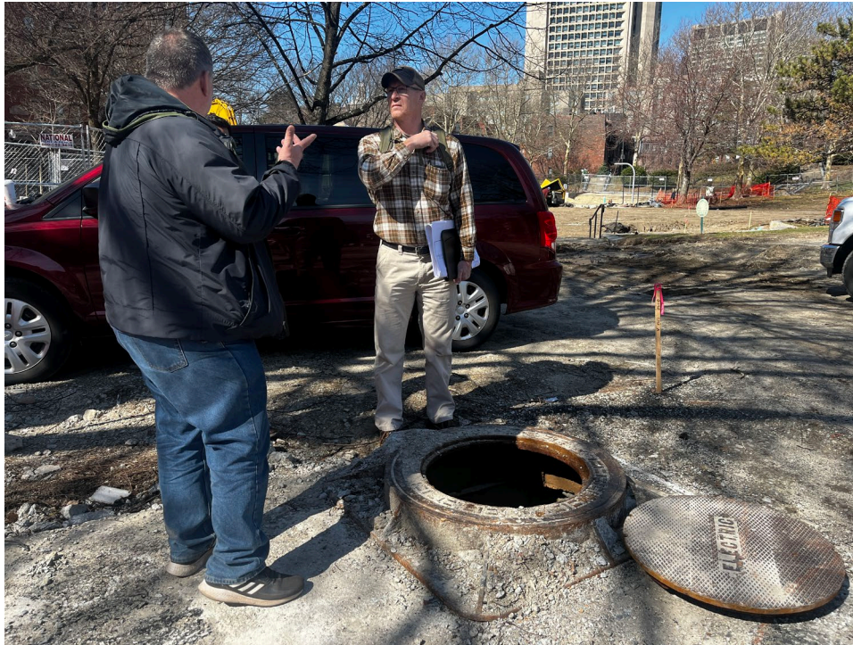
A large historic plumbing and electrical vault was discovered during demolition. The vault used to serve a fountain featured in the park 26 years ago.
