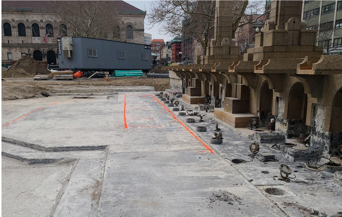
Now that we have encountered solid concrete in the main fountain basin, the contractor has sprayed orange lines where new pipes are going to be installed. Below the spouts, you can see where we've removed the base row of vertical stones to install new waterproofing behind them.
