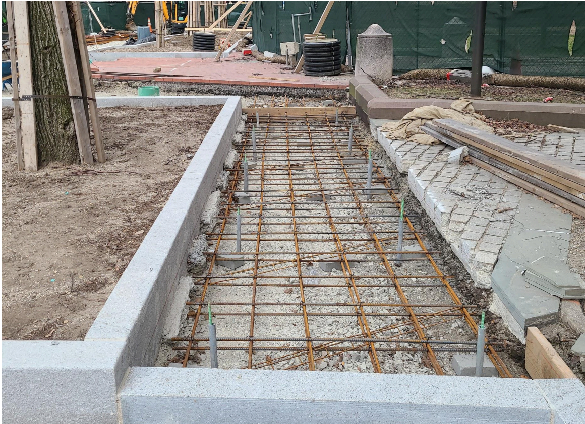
In the northeast “triangle,” between Trinity church and Boylston Street, we are ready for the temperature to be warm enough for concrete! Rebar awaits, adjacent to a new planter with an existing tree.
