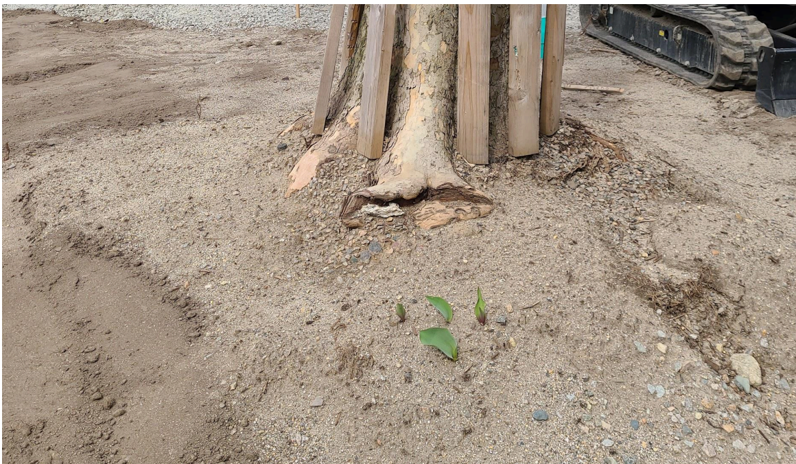
At the foot of an existing tree, despite all the construction mayhem, a tulip is poking through! Happy spring!
