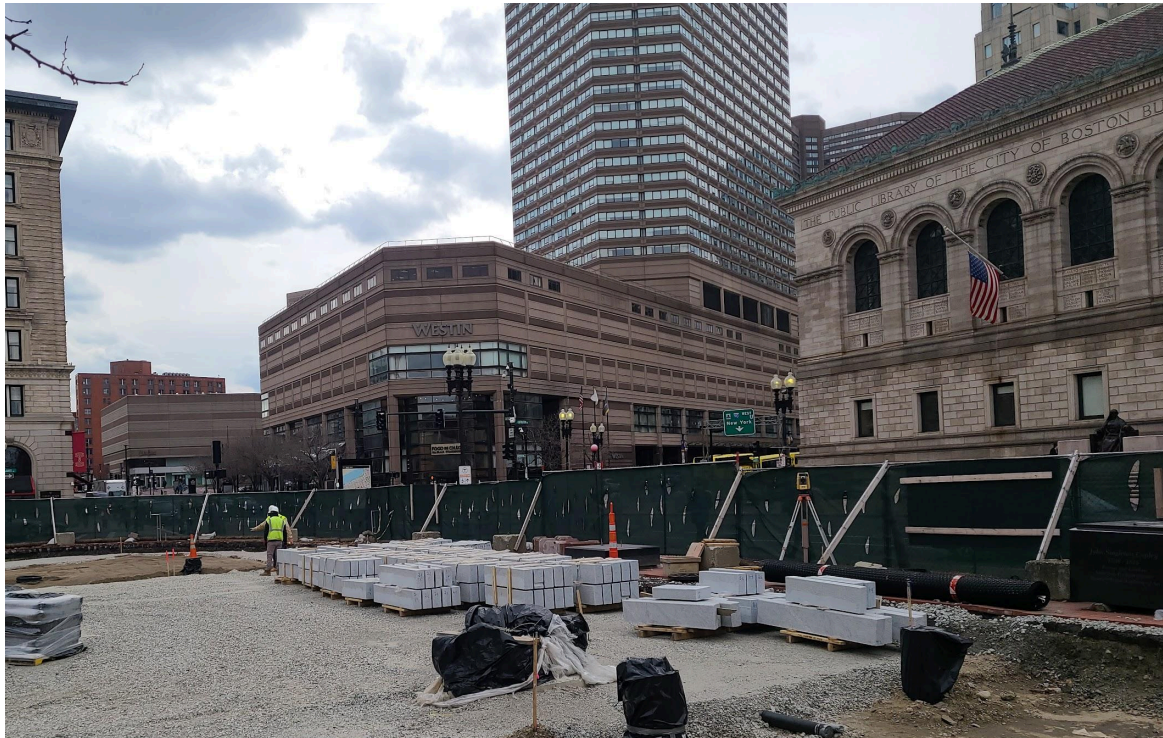
The remainder of the granite planter curbs, delivered to the site and waiting for installation. Each piece is labeled with the number of the planter, and where it goes within that planter.
