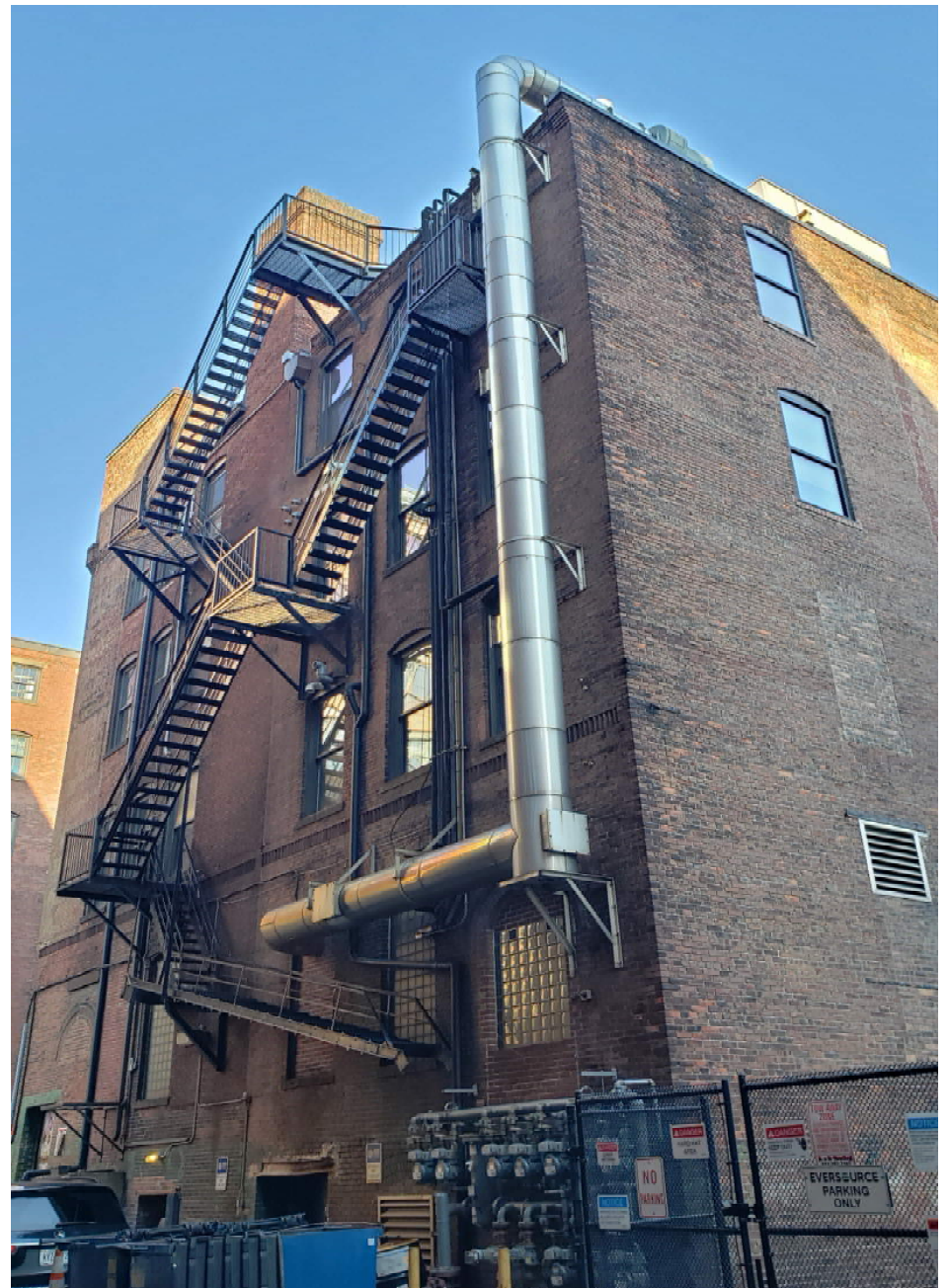
SURFACE MOUNTED DUCTWORK BEHIND "LUCKY'S"
