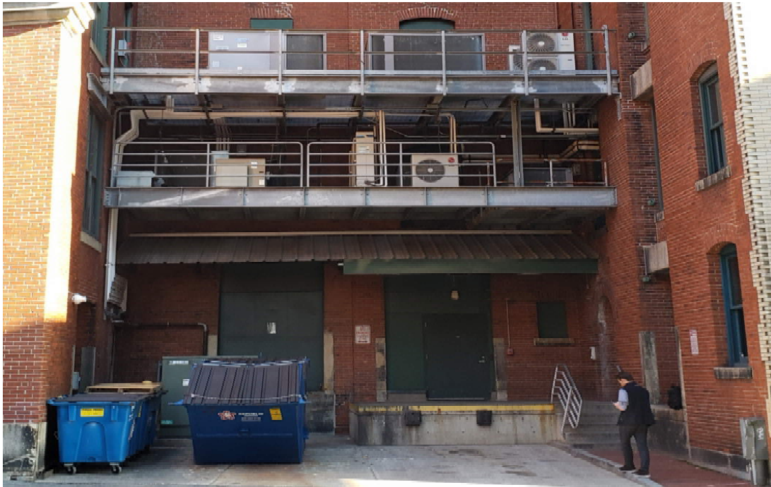
CONDENSERS BEHIND 281-283 SUMMER STREET
