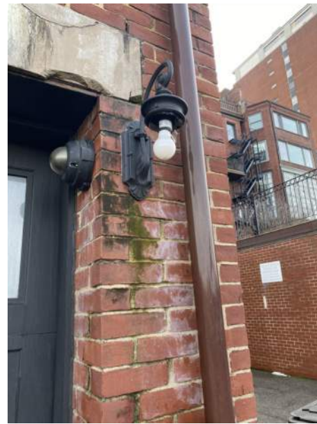
REPLACE BROKEN LIGHTS WITH NEW FIXTURES
