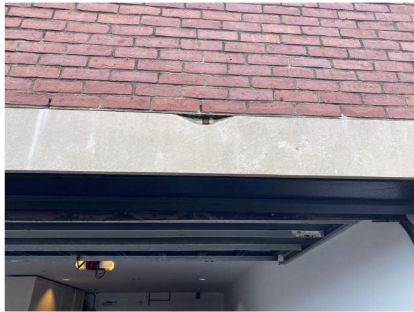
REPLACE CRACKED & CHIPPED LINTELS AT GARAGE
