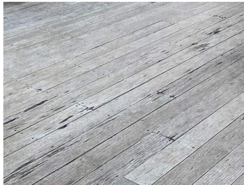
ROTTED DECK BOARDS
