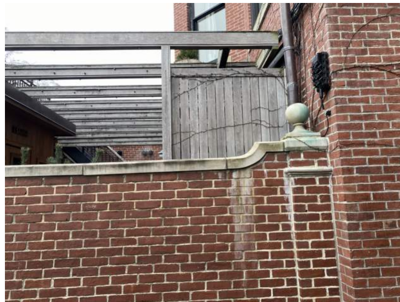
EXISTING STONE CAPS AT ALL LOCATIONS TO BE RESET WITH NEW WATERPROOFING & COPPER FLASHING
