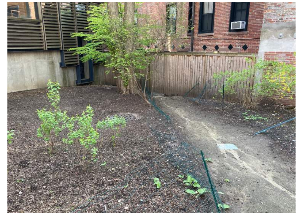
SLOPED GRADE ACROSS WATSON PARK CHANNELS STORM WATER INTO THE ADJACENT PROPERTY.
