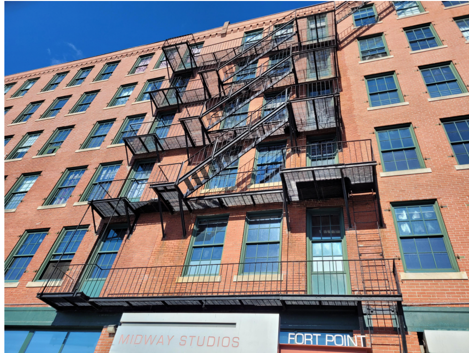
BACK ELEVATION - MEDALLION AVE EXISTING FIRE ESCAPE A (BETWEEN COLUMN LINES 5 AND 6) SEE SHEET A-202
