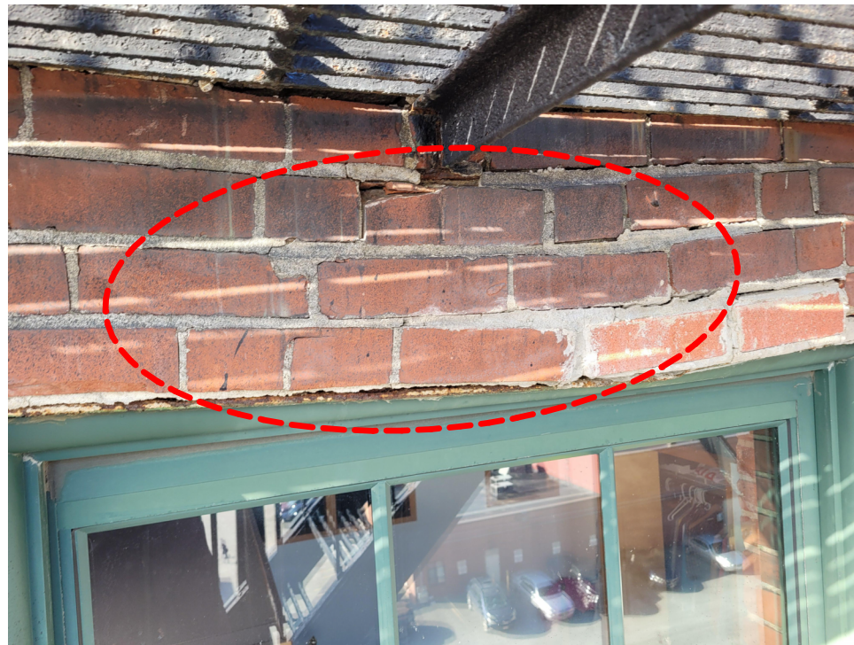
BRICK DISPLACEMENT AROUND THE WINDOW LINTEL. PORTION OF THE FIRE ESCAPE LANDING IS BEING SUPPORTED BY THIS DETERIORATED SOLID MASONRY WALL AREA.
