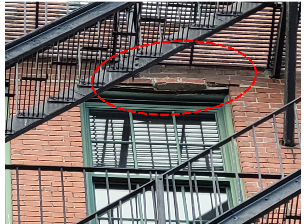
SIGNIFICANT MOVEMENT OF THE BRICK AROUND THE WINDOW LINTEL. PORTION OF THE FIRE ESCAPE LANDING IS BEING SUPPORTED BY THIS DETERIORATED SOLID MASONRY WALL AREA.
