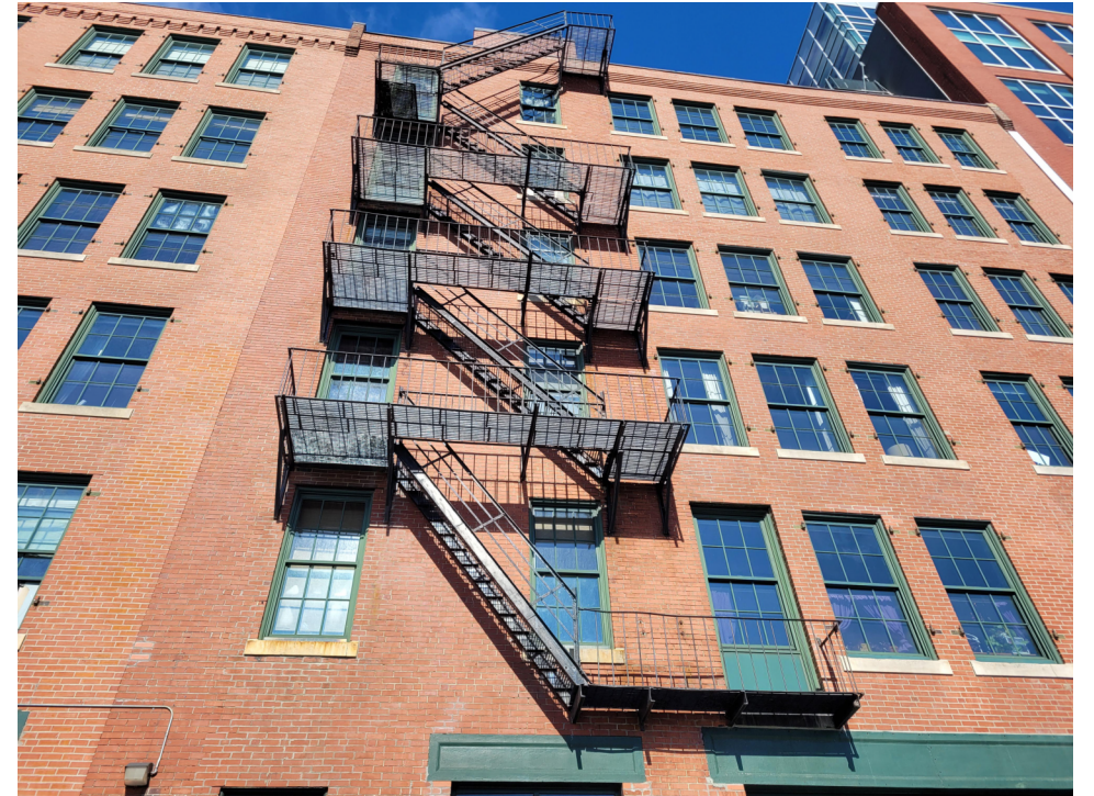
BACK ELEVATION - MEDALLION AVE EXISTING FIRE ESCAPE B (BETWEEN COLUMN LINES 9 AND 10) SEE SHEET A-203
