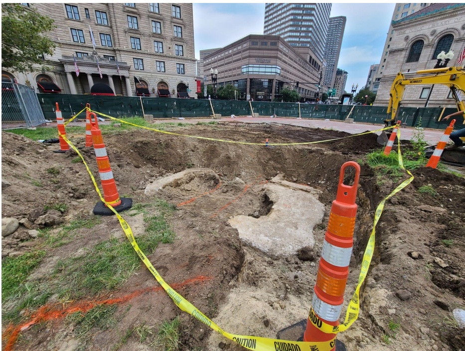
An old drainage vault below Huntington Avenue. Our test pit revealed it's true location was shallower and about 10' north of where we thought. The civil engineer redesigned much of the drainage as a result. We will fill it so it doesn't collapse in the future!
