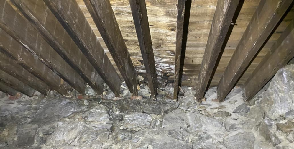
SEVERLY ERODED FRAMING
