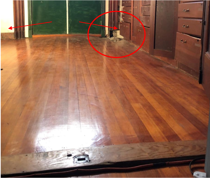
PARTIALLY COLLAPSING FLOOR
