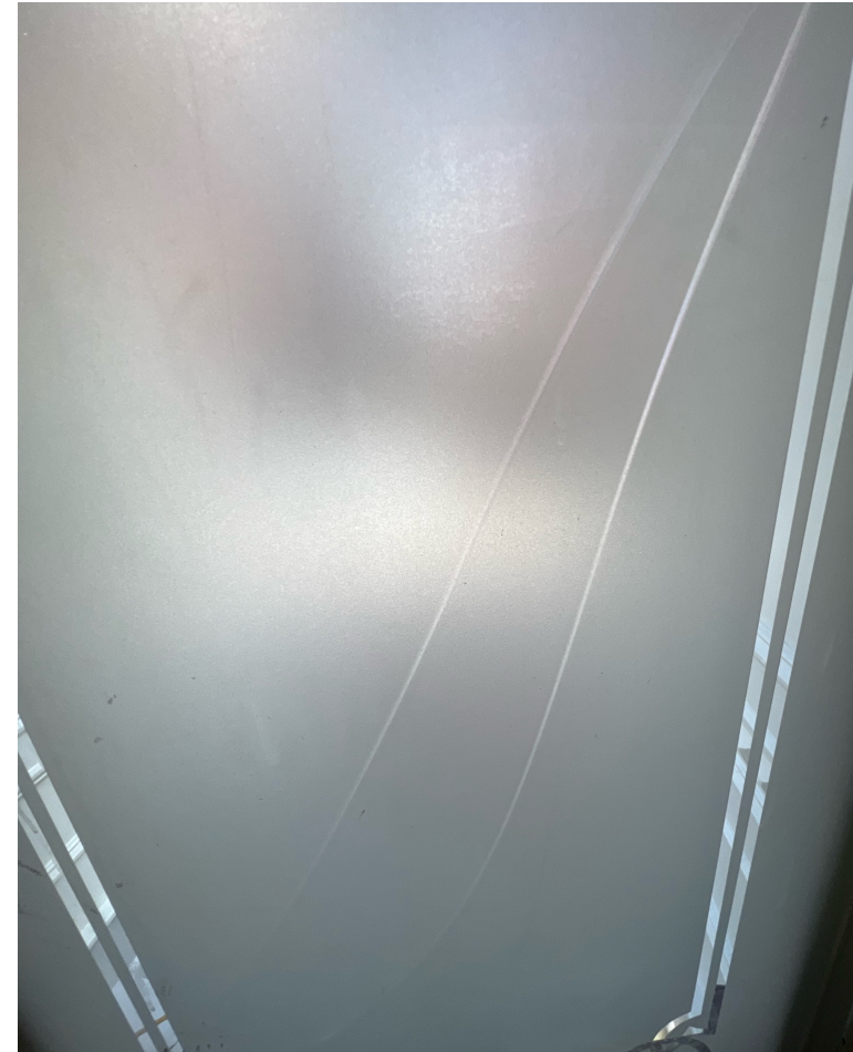
Broken Panel Close Up
