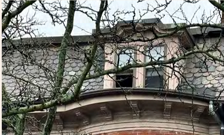
Existing mansard shingles to be replaced with like-kind composite shingles to match
