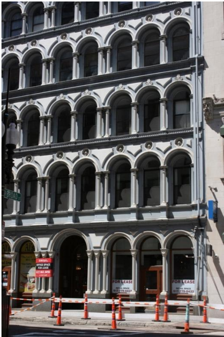
Figure 3. State Street façade; detail of 1st – 4th floors, east side of building.
