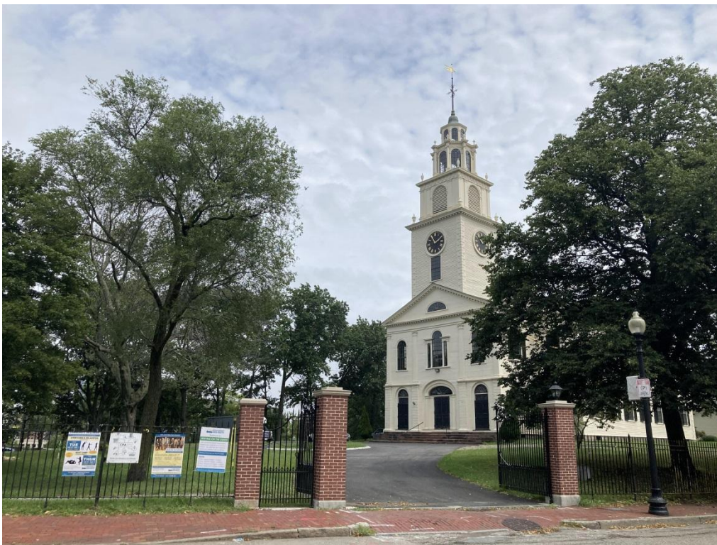
Figure 11. Gateway at Dudley Street entrance, after being widened to accommodate emergency vehicle access; historic cast iron gates restored. August 2021.
