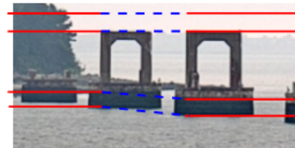
Approximate bottom of steel elevation Top of pier bolster Approximate high tide elevation Approximate low tide elevation
