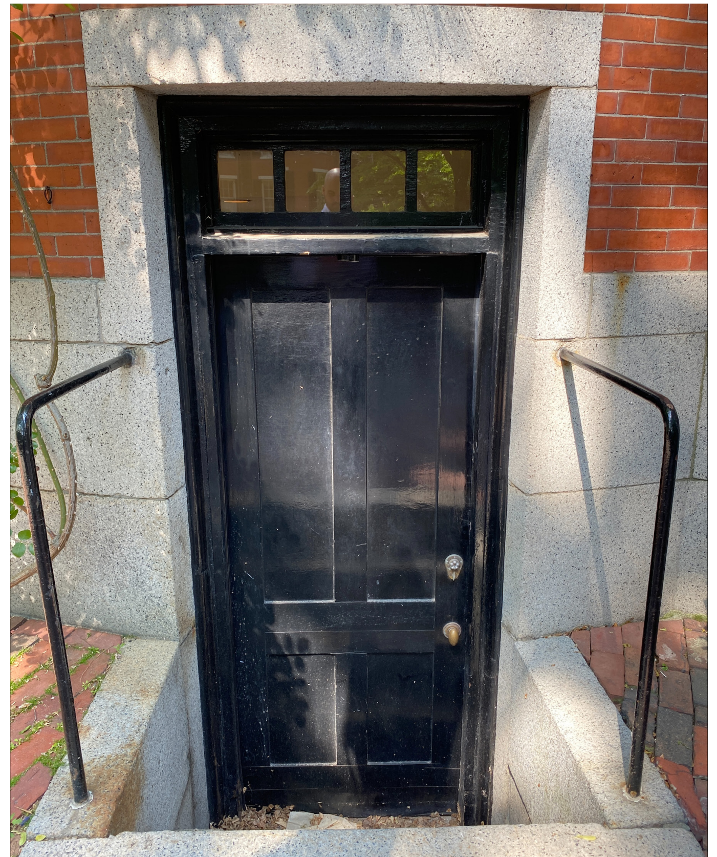
Lower Level Door - Full replacement of door, transom and trim to match existing.
