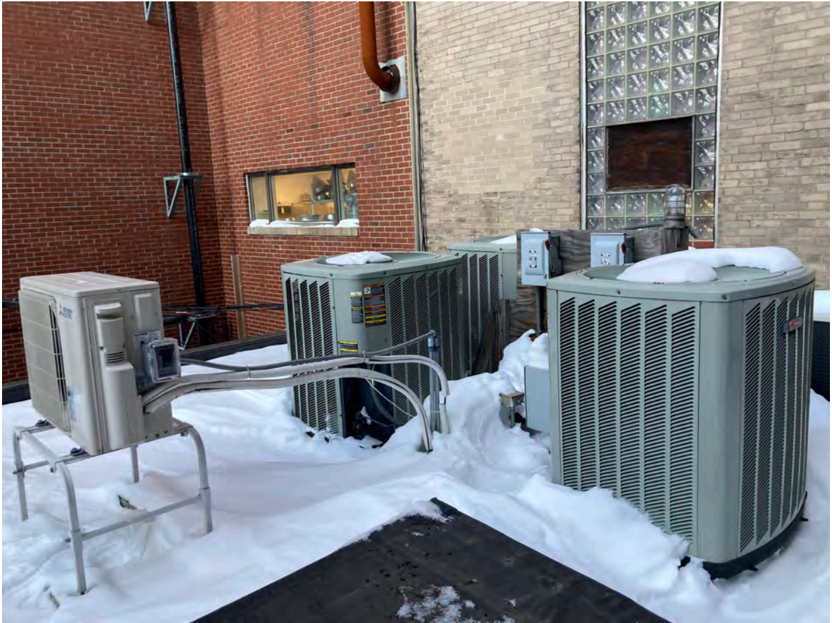
7 - 9 Newbury Street Rear Alley Roof Existing Compressors
