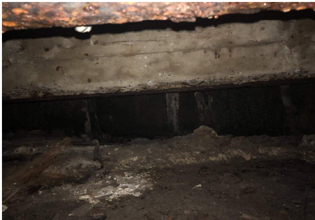
Photograph No. 6: View beneath cast-in-place slab of void exposing granite block wall face.
