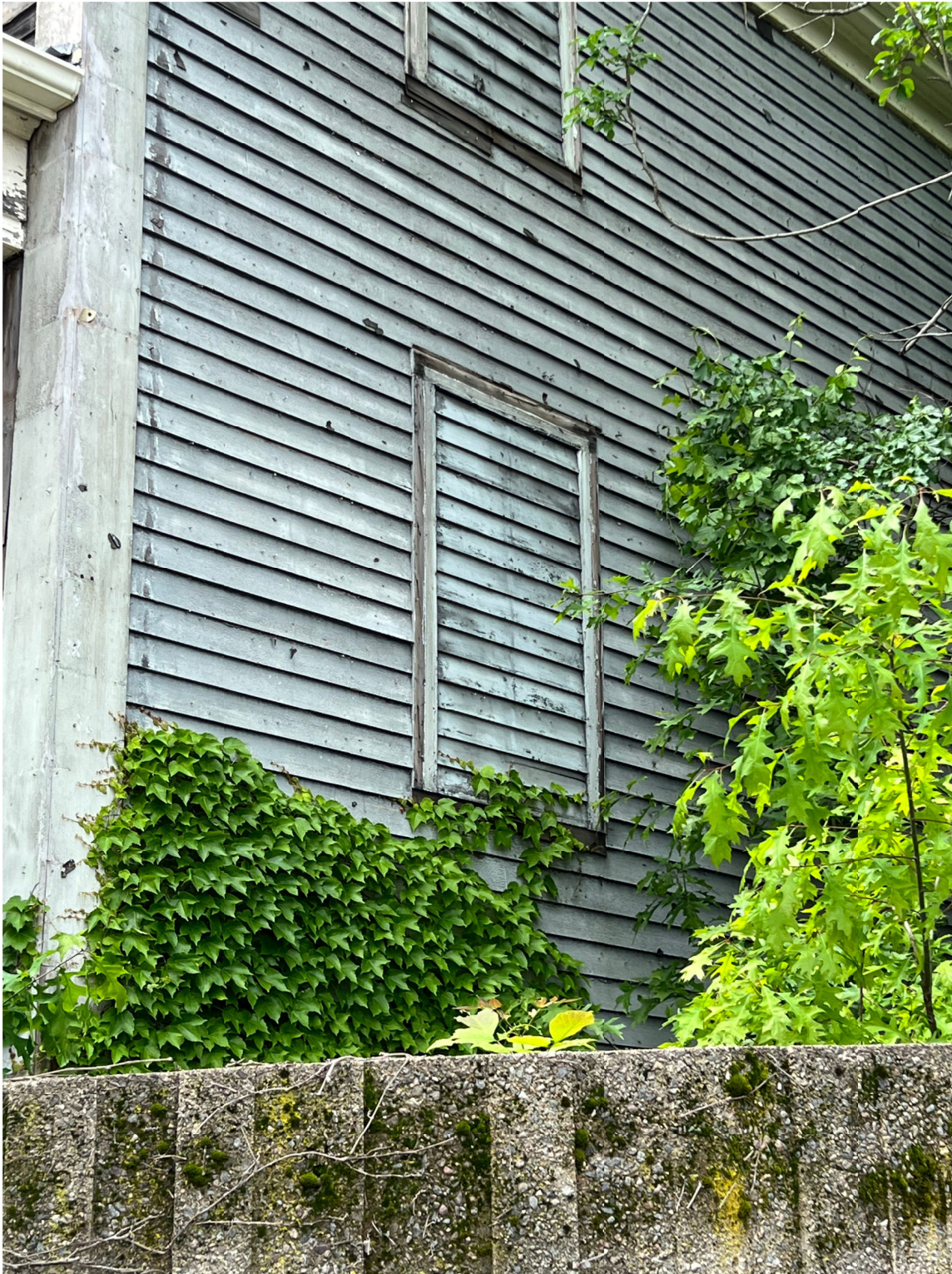
Figure 14. North elevation with first- and second-floor windows removed and covered with siding. Taken June 2, 2022.
