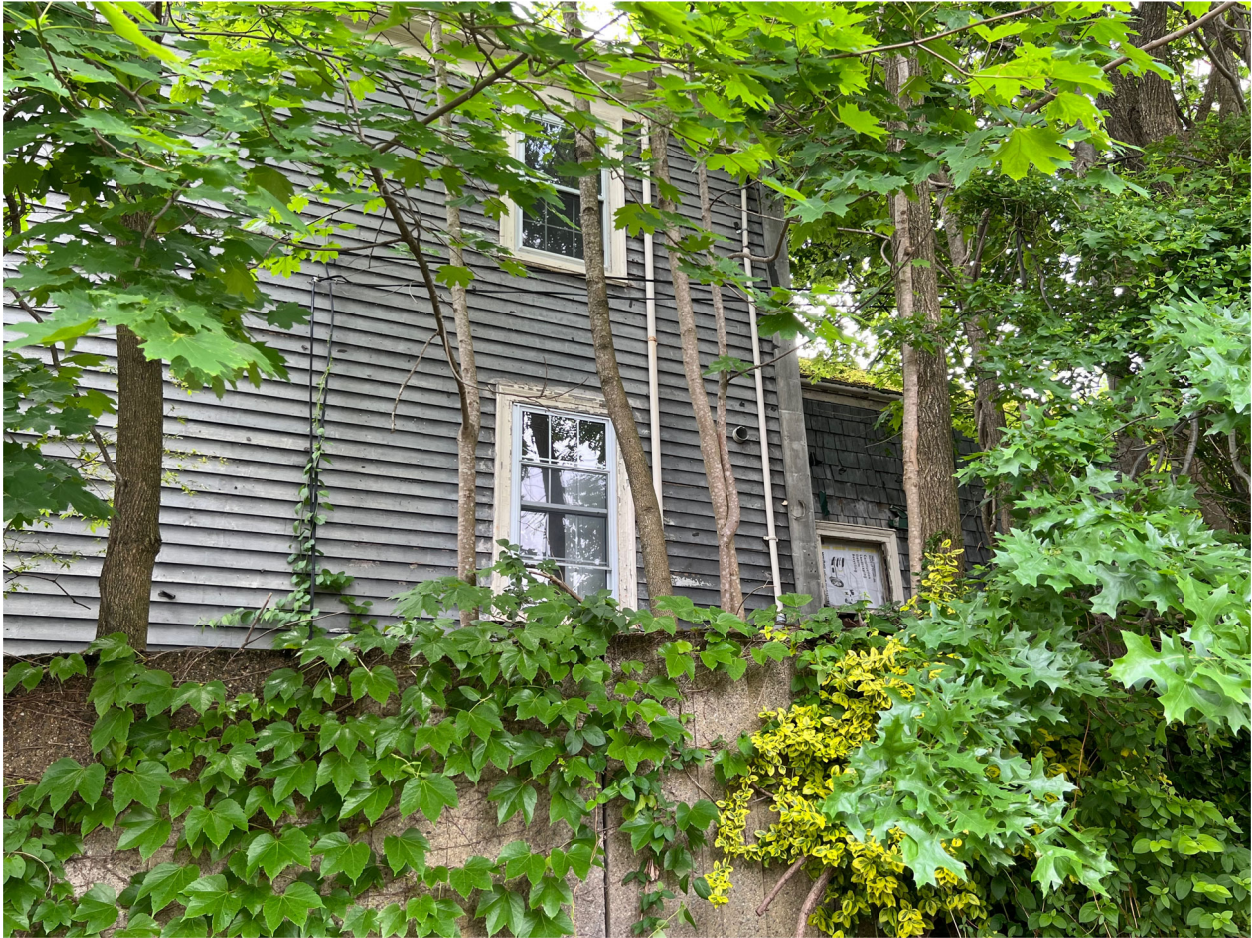
Figure 15. Two windows on north elevation toward rear of the house, taken on June 2, 2022. The missing window on the side of the ell is partially visible.
