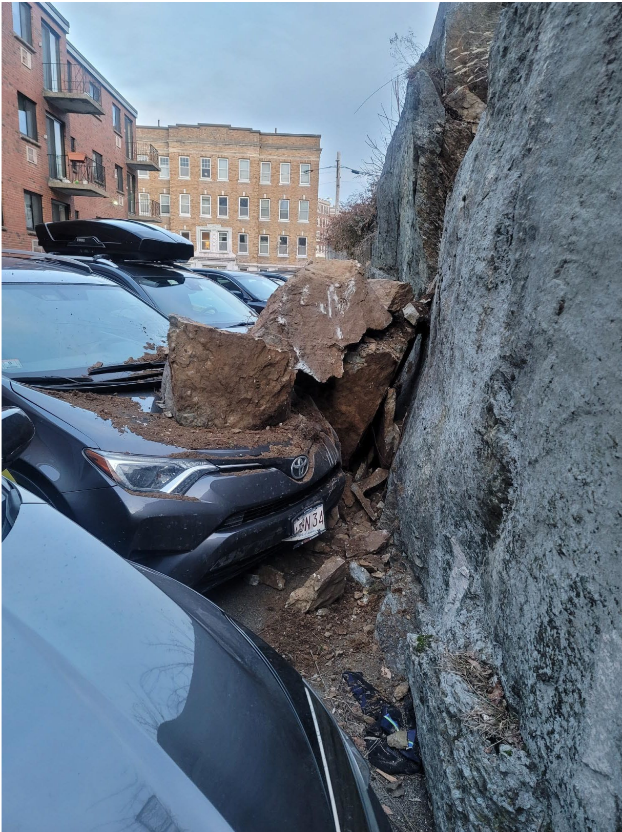
Photo #3 – March 15, 2022 Collapse Area and Impact to Cars Beneath
