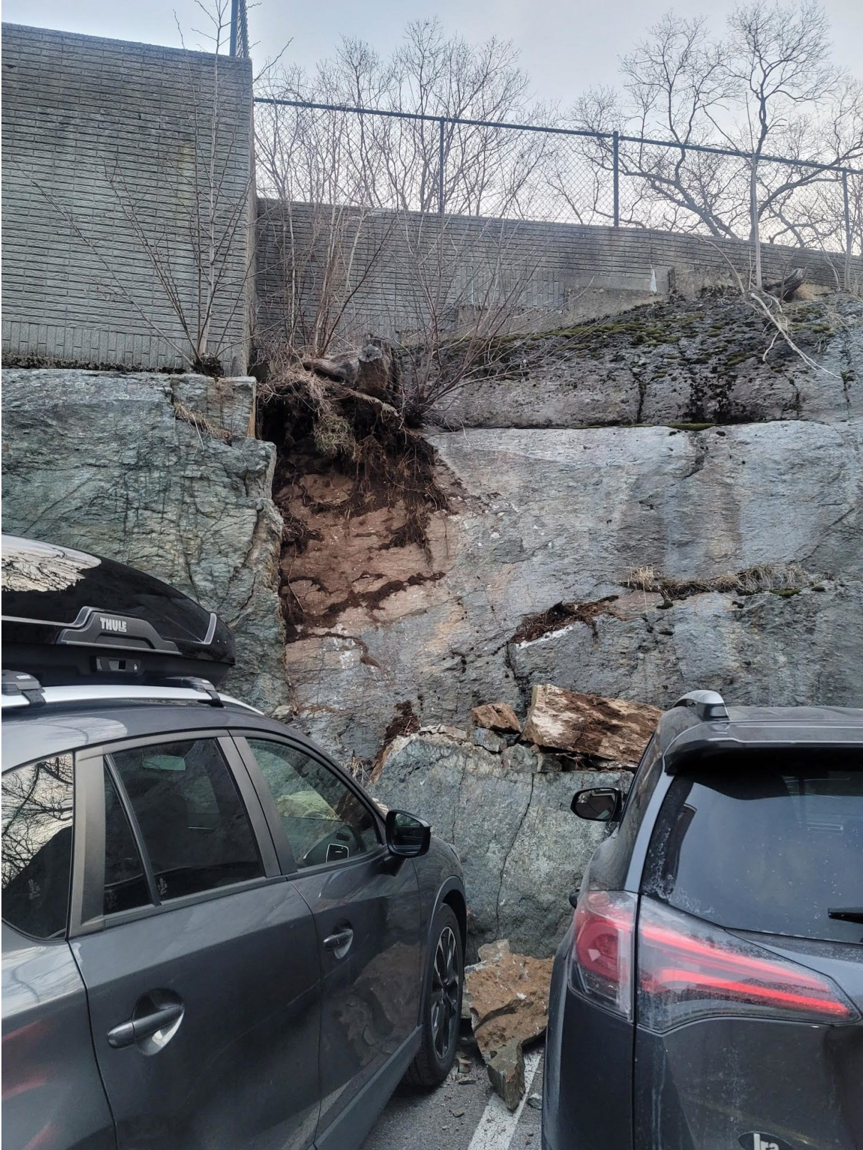
Photo #4 – March 15, 2022 Collapse Area and Impact to Cars Beneath
