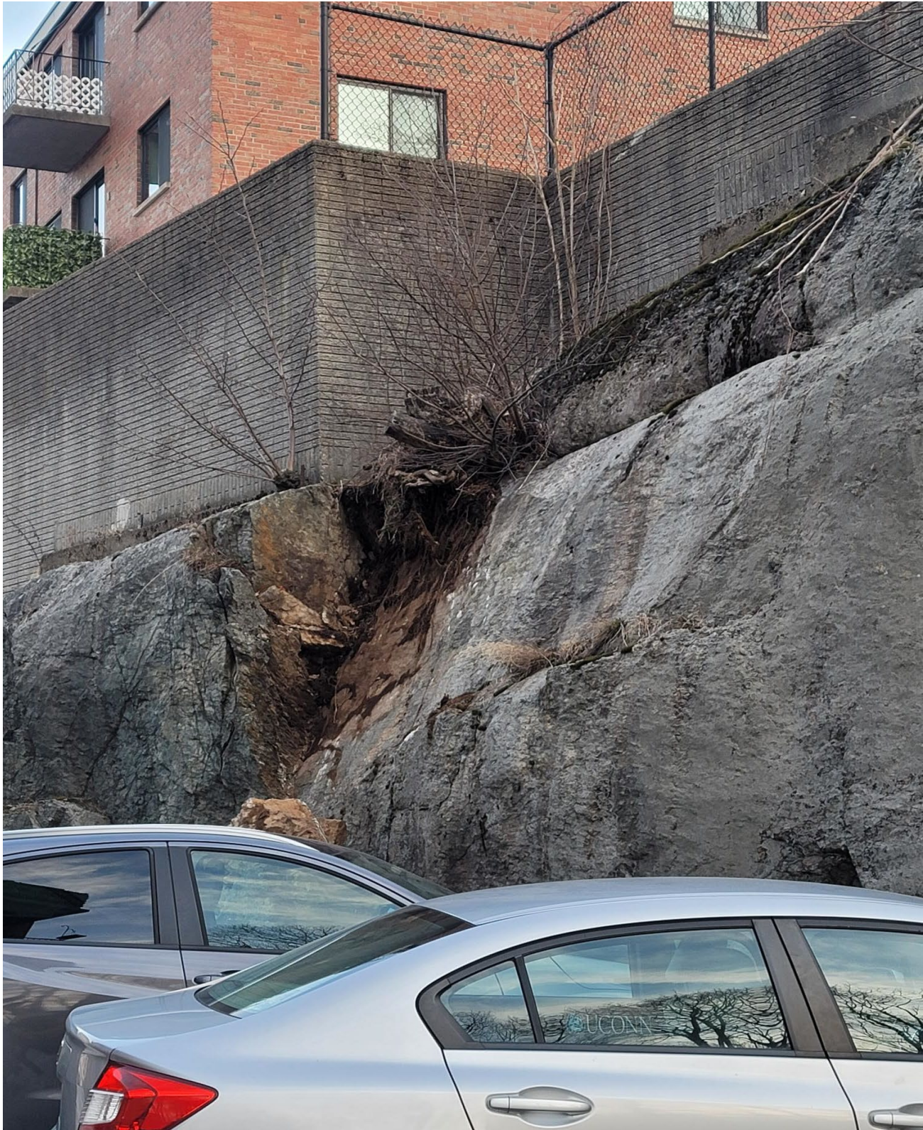
Photo #1 – March 15, 2022 Collapse Area
