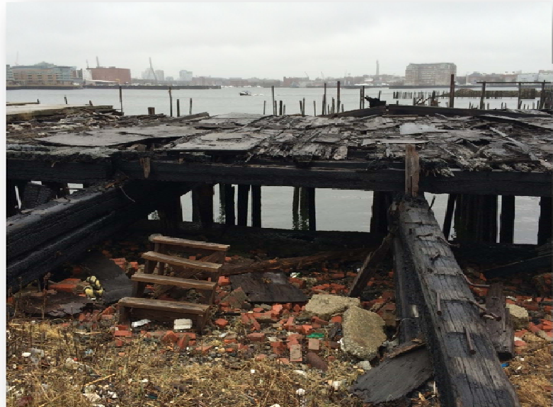
Figure 2, Existing Conditions. The existing condition of Clippership Wharf showing areas of abandoned and degraded dock and pilings and various debris.
