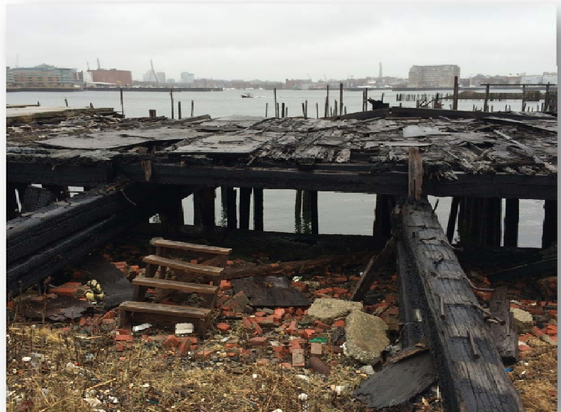
Figure 2, Existing Conditions. The existing condition of Clippership Wharf showing areas of abandoned and degraded dock and pilings and various debris.
