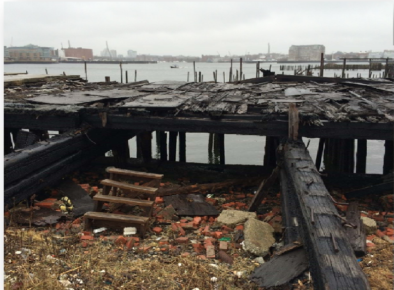
Figure 2, Existing Conditions. The existing condition of Clippership Wharf showing areas of abandoned and degraded dock and pilings and various debris.
