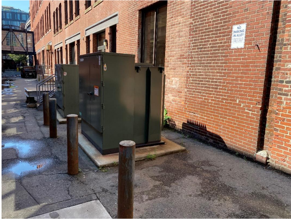
Picture 3: Transformer pad and electrical equipment in private alley way behind building.
