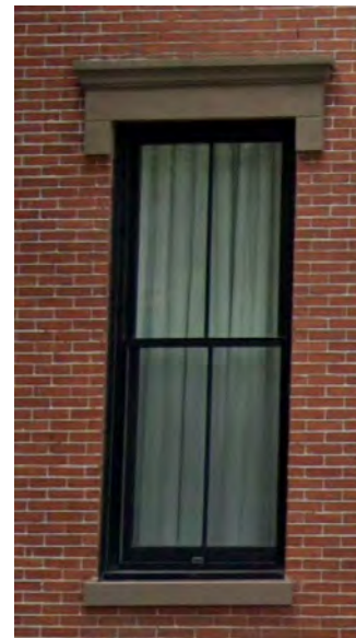
Existing window on Level 2 Paint color on windows, sills, and lintels to match
