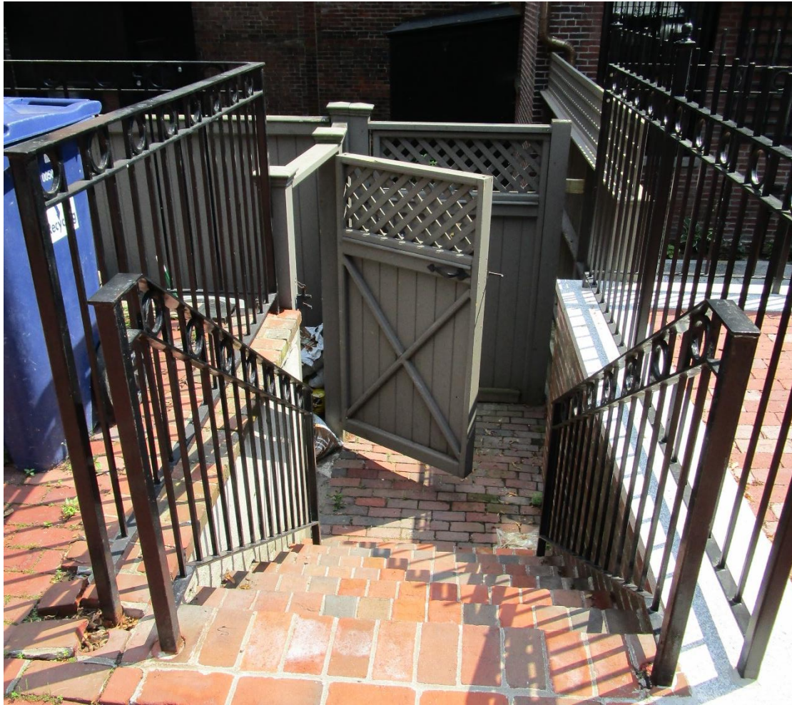
View of existing modern metal handrails at rear of property, new handrails match detailing
