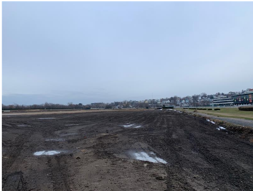
View looking northwest across infield Central Common grading work towards grandstand building. Photograph dated January 14, 2022.
