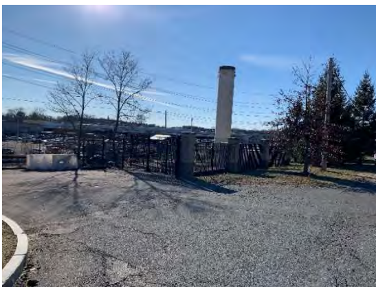
Photograph #17 Enclosed landfill gas flare system.
