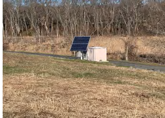
Photograph # 16 Solar condensate pump enclosure on at the foot of the northeastern sieslope.
