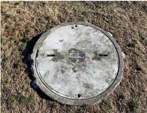
Photograph #17 Fiberglass landfill gas system well vault.
