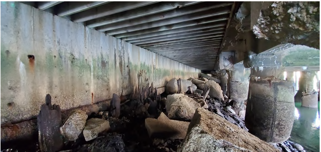
Photo 2: Overall view of timber stringers on top of the undermined seawall.
