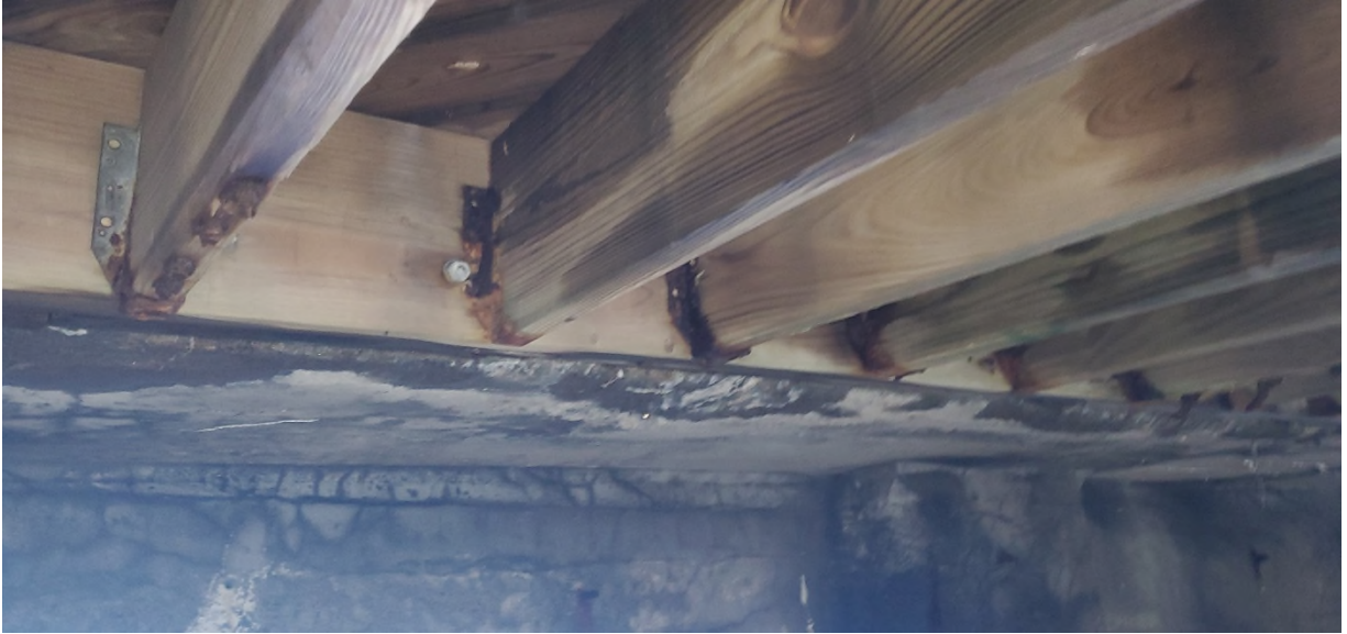
Photo 3: Deteriorated stringer hangers.
