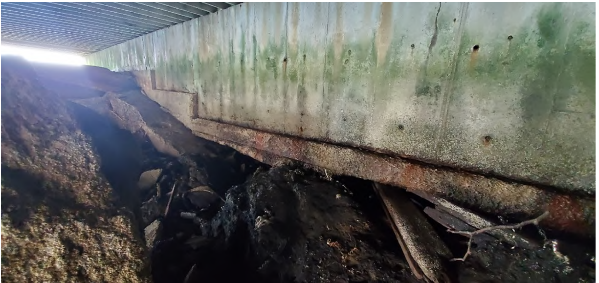
Photo 4: Typical undermining of the seawall.
