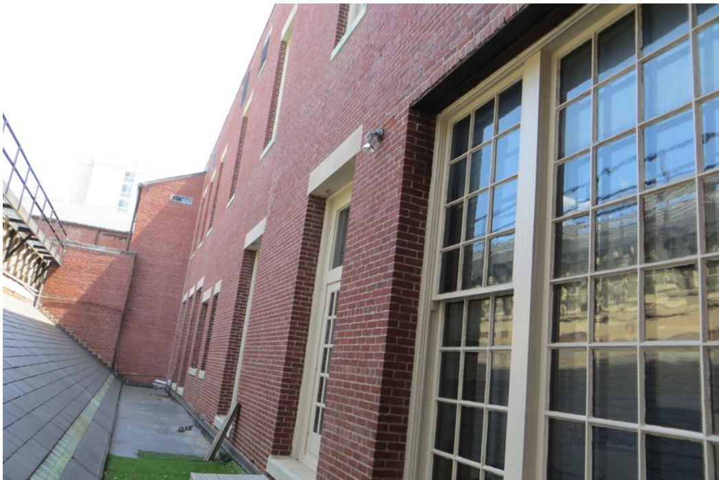
Figure #11. East elevation second story and attic level windows (from first story roof, looking south). July 2016.
