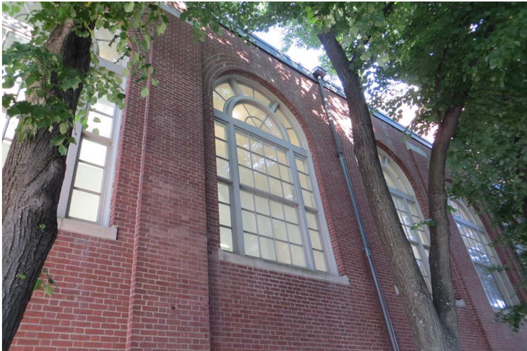
Figure #10. Windows on the one-story section of east elevation (looking west). June 2016.
