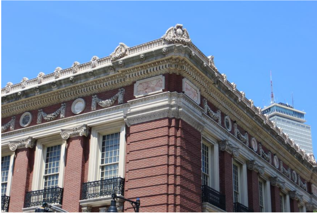
Figure #5. Entablature and cheneau at the corner of south and west facades (looking northeast). July 2016.
