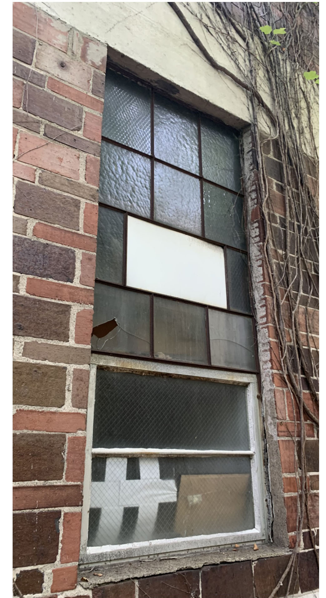
Typical irreparable damaged steel window to be replaced
