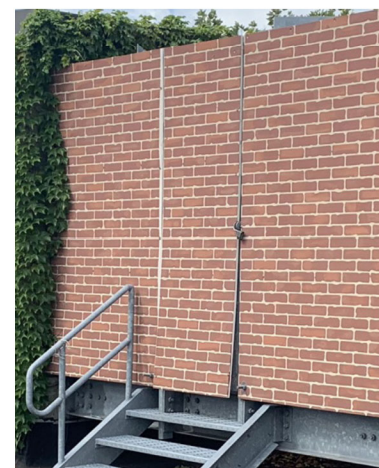
Existing faux brick to be replaced
