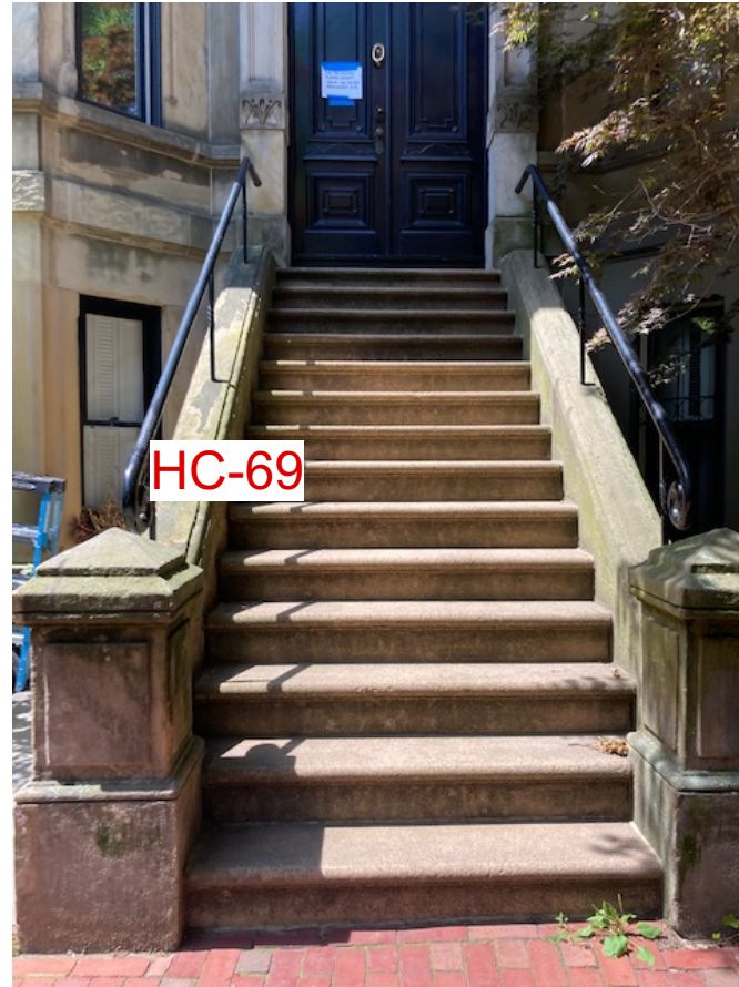
#26 HOLYOKE STREET EXISTING FRONT STEPS TO BE REFINISHED AND MATCHED EXACTLY TO THE ADJACENT HOUSES (#24 / #28)
