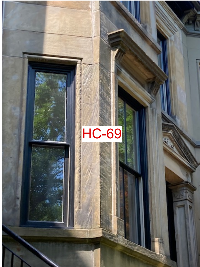
#26 HOLYOKE STREET EXISTING FACADE / WINDOWS CONDITION.
