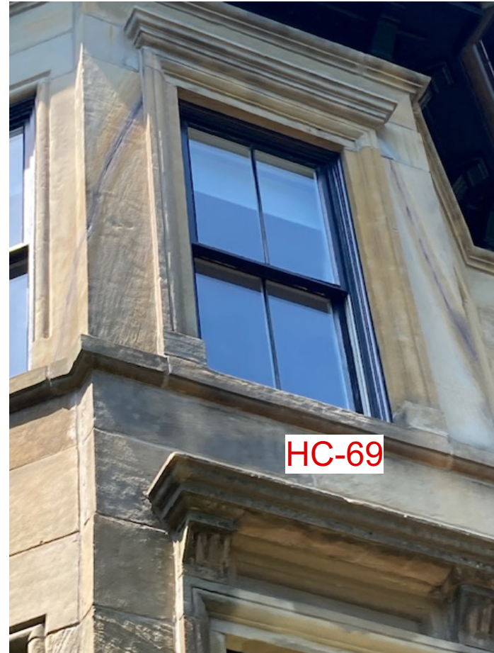
#26 HOLYOKE STREET EXISTING FACADE / WINDOWS CONDITION.
