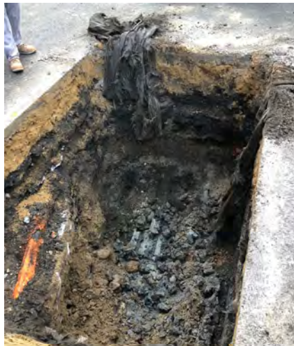
Photo 22: View looking into HA19-TP6; concrete duct bank exposed at northeast end of test pit
