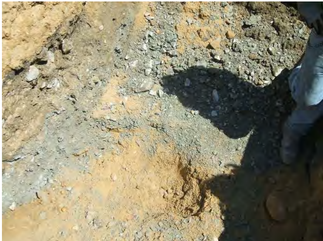
Photo 19: Top of tunnel protective slab encountered depth of 4.6 ft below existing site grades at HA19-TP5
