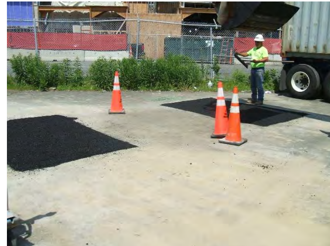
Photo 8: Asphalt patch at HA19-TP2 and HA19-TP3
