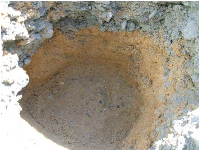
Photo 3: Hand excavated to top of tunnel protective slab at depth of 4.4 ft below existing site grades at HA19-TP1
