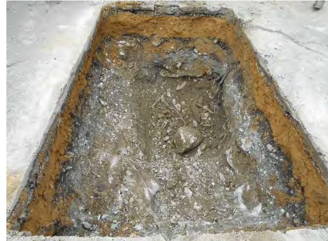
Photo 25: Dense graded material and concrete rubble/debris encountered at depth of approx. 1.9 ft below existing grades at HA19-TP7
