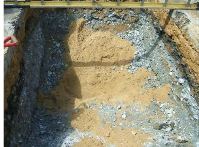
Photo 14: Looking into HA19-TP4 excavation; hand excavated to top of tunnel protective slab at depth of 4.8 ft below existing site grades
