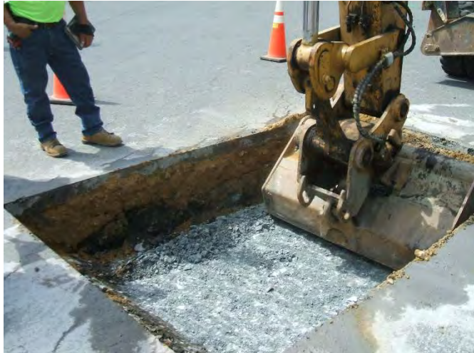
Photo 13: View looking south at HA19-TP4
