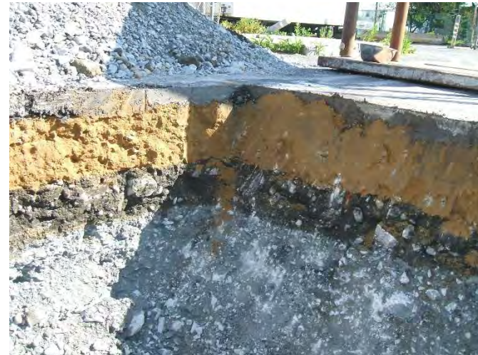
Photo 33: Typical cross-section of fill material placed over CA/T tunnel alignment at HA19-TP9
