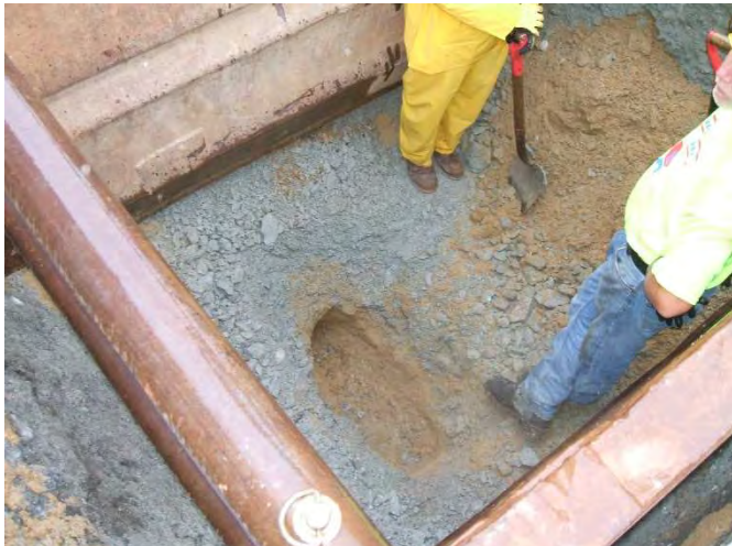
Photo 11: Hand excavated at HA19-TP3 to top of tunnel protective slab at depth of 7.9 ft below existing site grades
