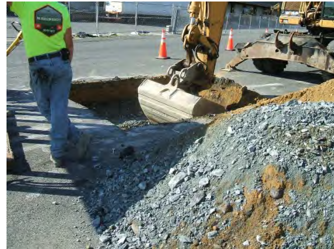
Photo 28: Excavating at HA19-TP8, located near the center of the I-90 CA/T tunnel alignment
