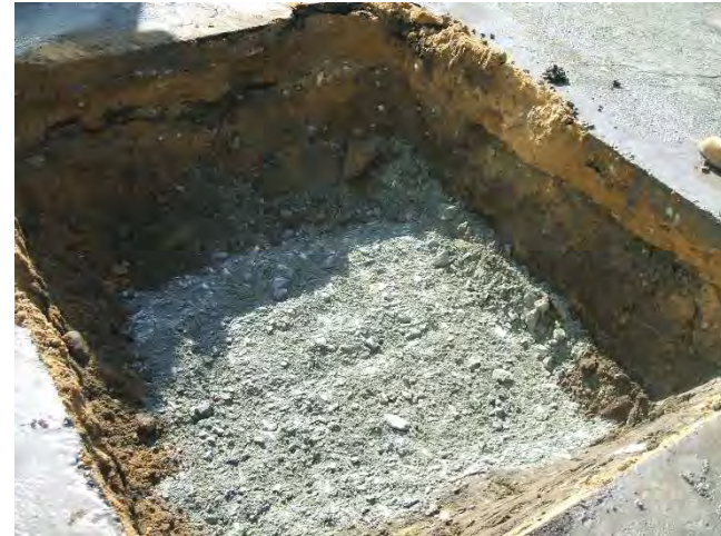
Photo 2: Dense graded fill encountered at depth of approx. 2 ft below existing site grades at HA19-TP1
