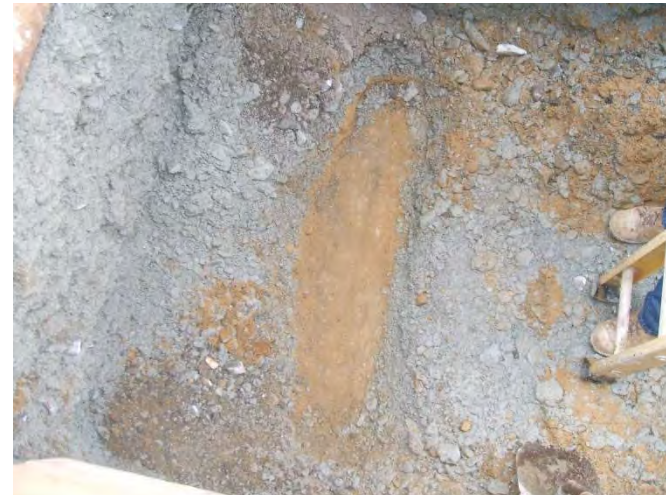
Photo 31: Hand excavated to top of tunnel protective slab at depth of 6.0 to 6.5 ft below existing site grades at HA19-TP8
