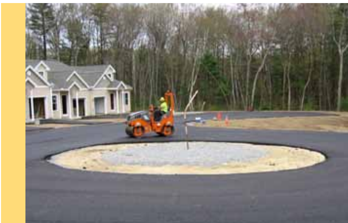
Final rolling of a new porous asphalt roadway installation in a residential subdivision in NH.
