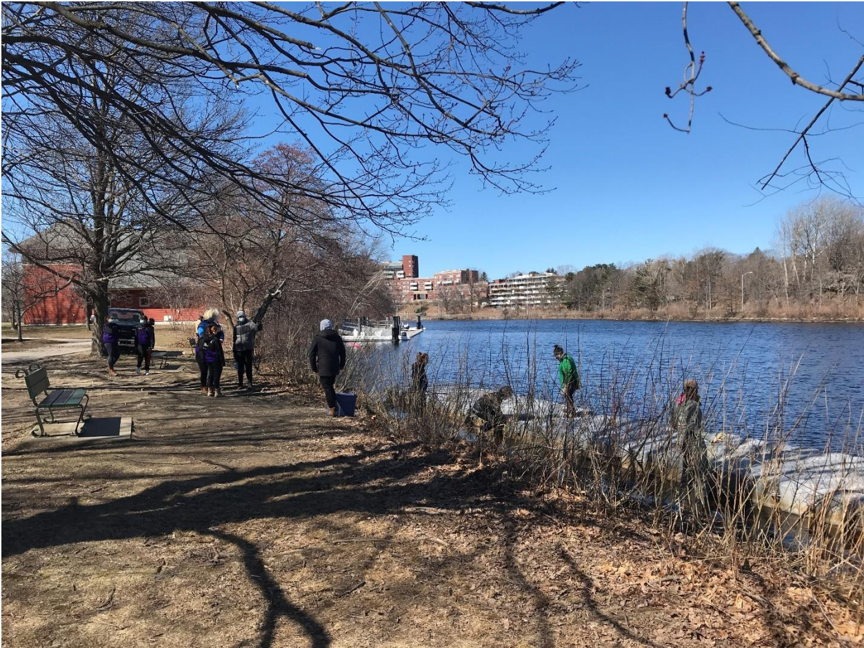
Photo of temporary dock during installation looking upstream to the Henderson Boat House:
