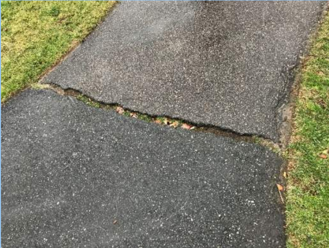
Upper Pathway Cracking
