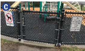
Settled Pathways & Damaged Gate
