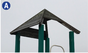
Damaged Playground Roof
