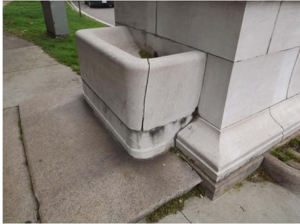
PHOTO SHOWING CRACK IN SOUTH BASIN (PRE 2017 CONDITION)
