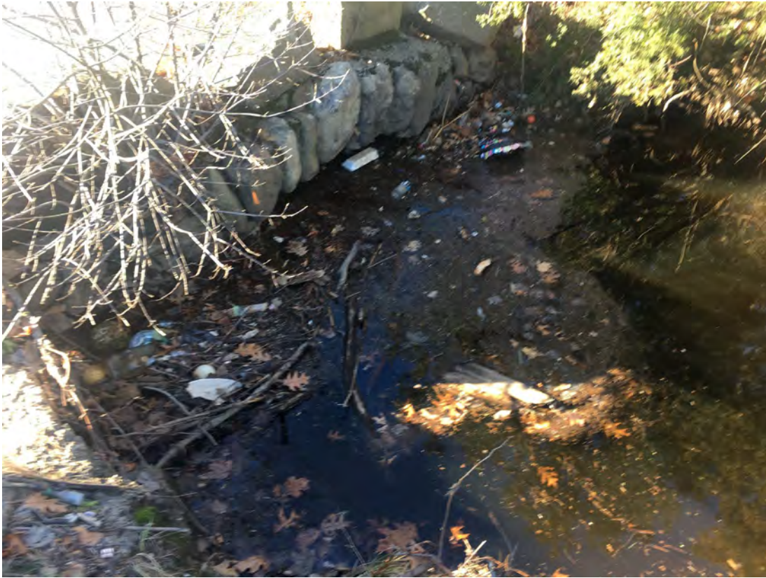
STR1: Debris Upstream of Headwall to be Removed
