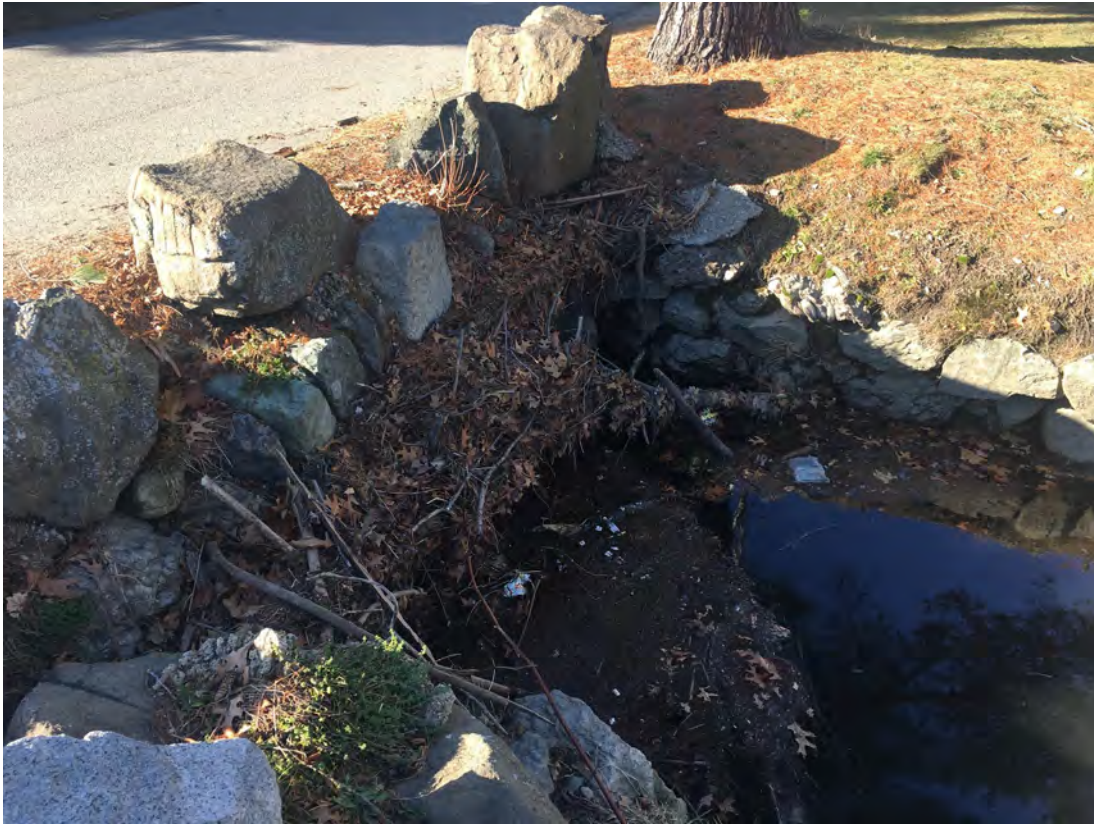
STR3: Branches and Debris Upstream of Headwall to be Removed
