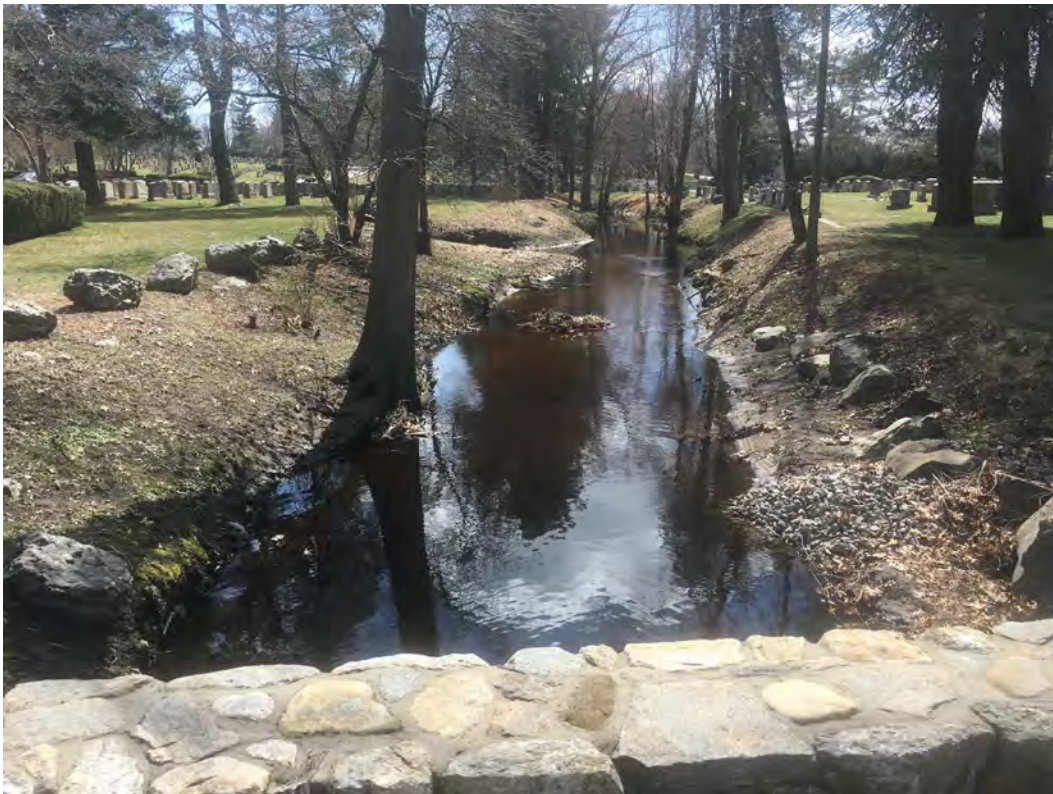
View Downstream from Third Crossing showing Debris and Rip Rap
