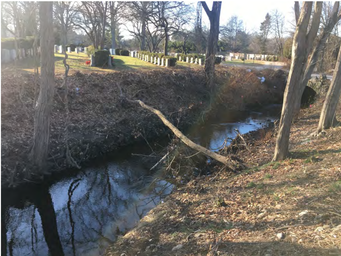
STR8: Log over Stream and Debris in Stream to be Removed
