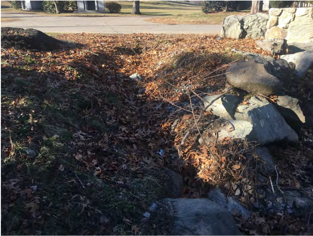
RRP1: Eroded Rip-Rap to be Replaced
