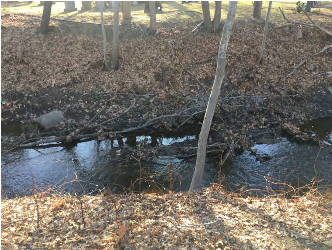
STR6: Branches and Debris to be Removed
