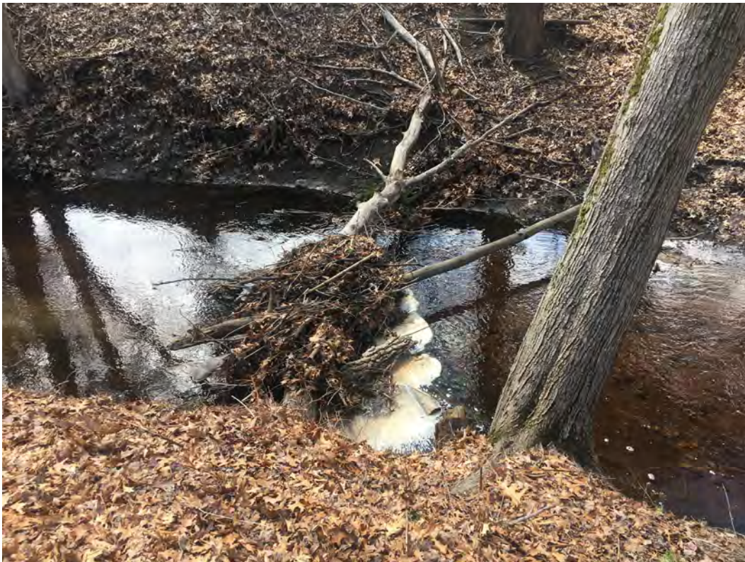
View of Log and Debris Dam Downstream of First Crossing
