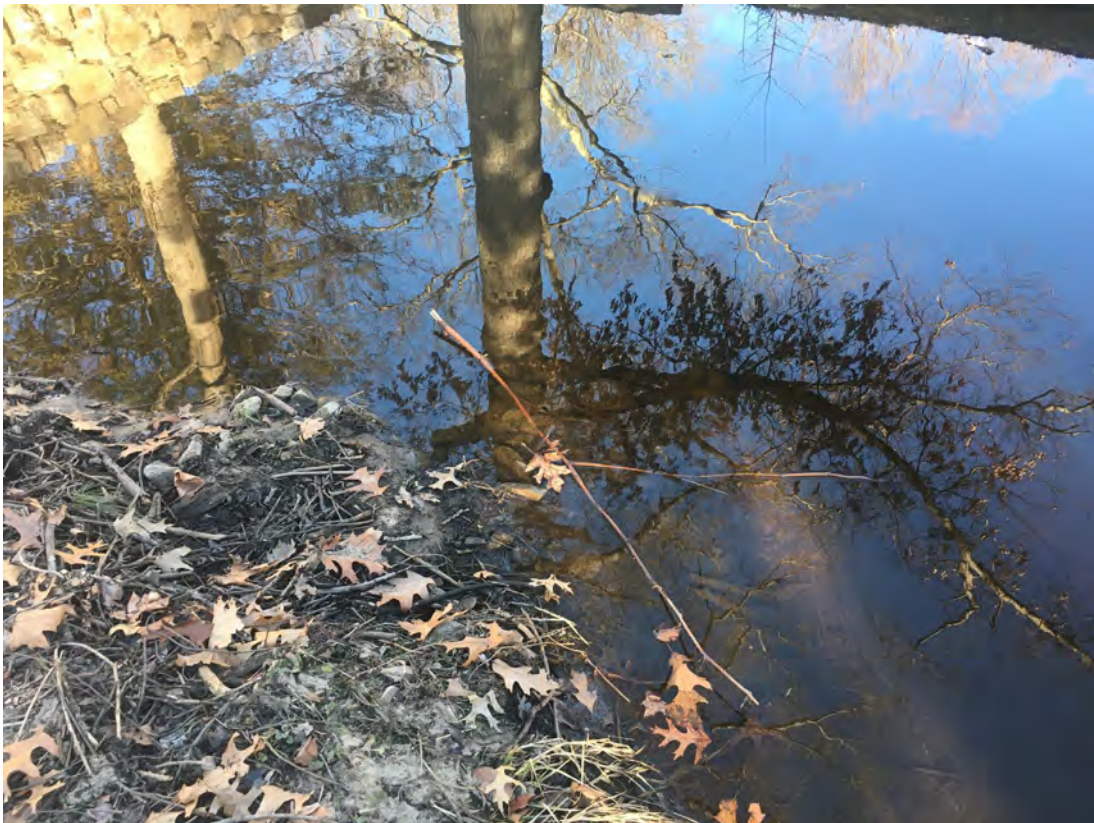
RRP2: Eroded Rip-Rap to be Removed from Stream
