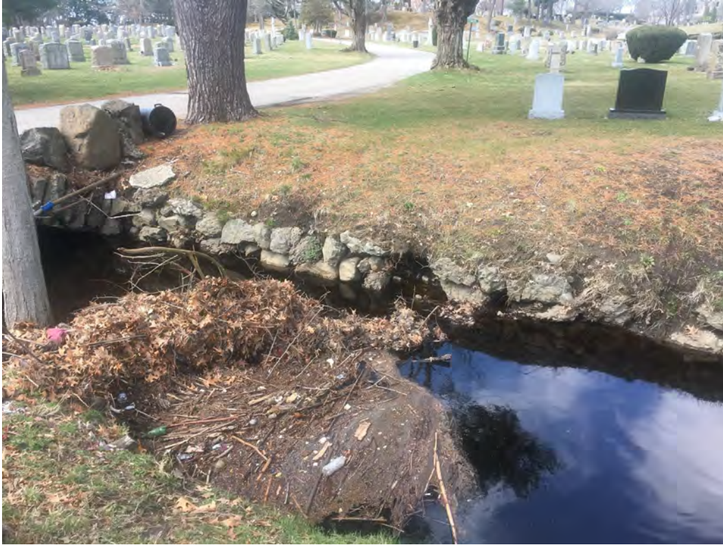
Debris Dam Located Upstream of Fourth Crossing
