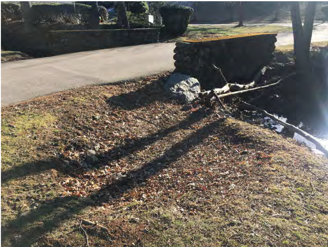
RRP3: Rip-Rap to be Removed and Replaced
