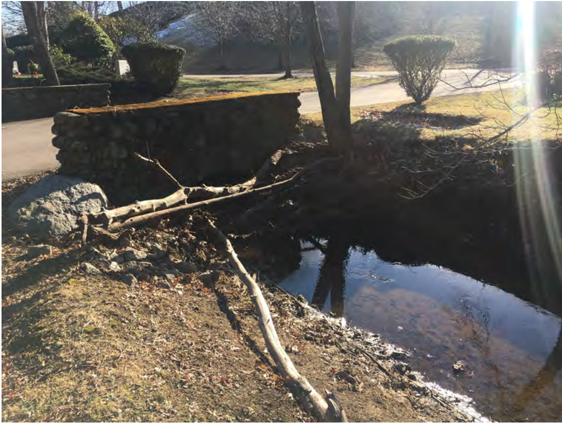
STR5: Logs and Debris Upstream of Headwall to be Removed
