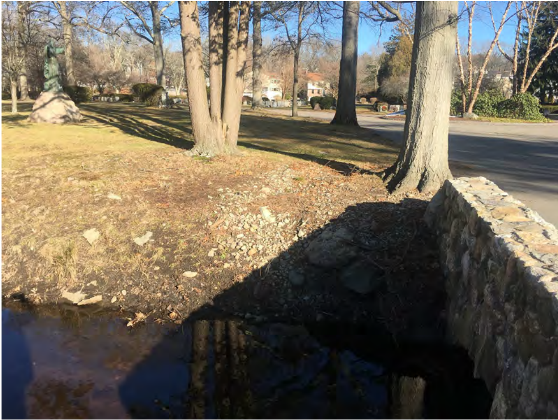
RRP2: Rip-Rap to be Removed and Replaced
