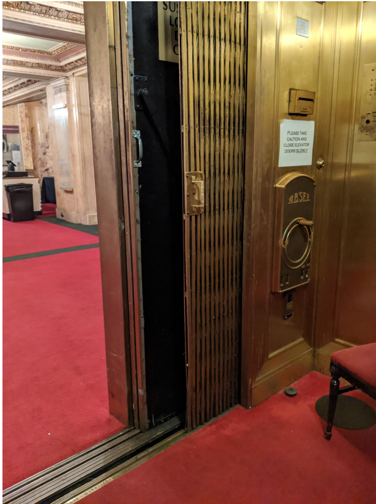
Elevator Cab Interior Showing Cage Door and Manual Operator
