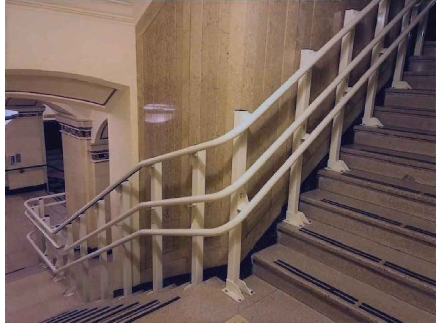
Portion of Stair Lift to be Removed and Handrail to Match Existing Provided
