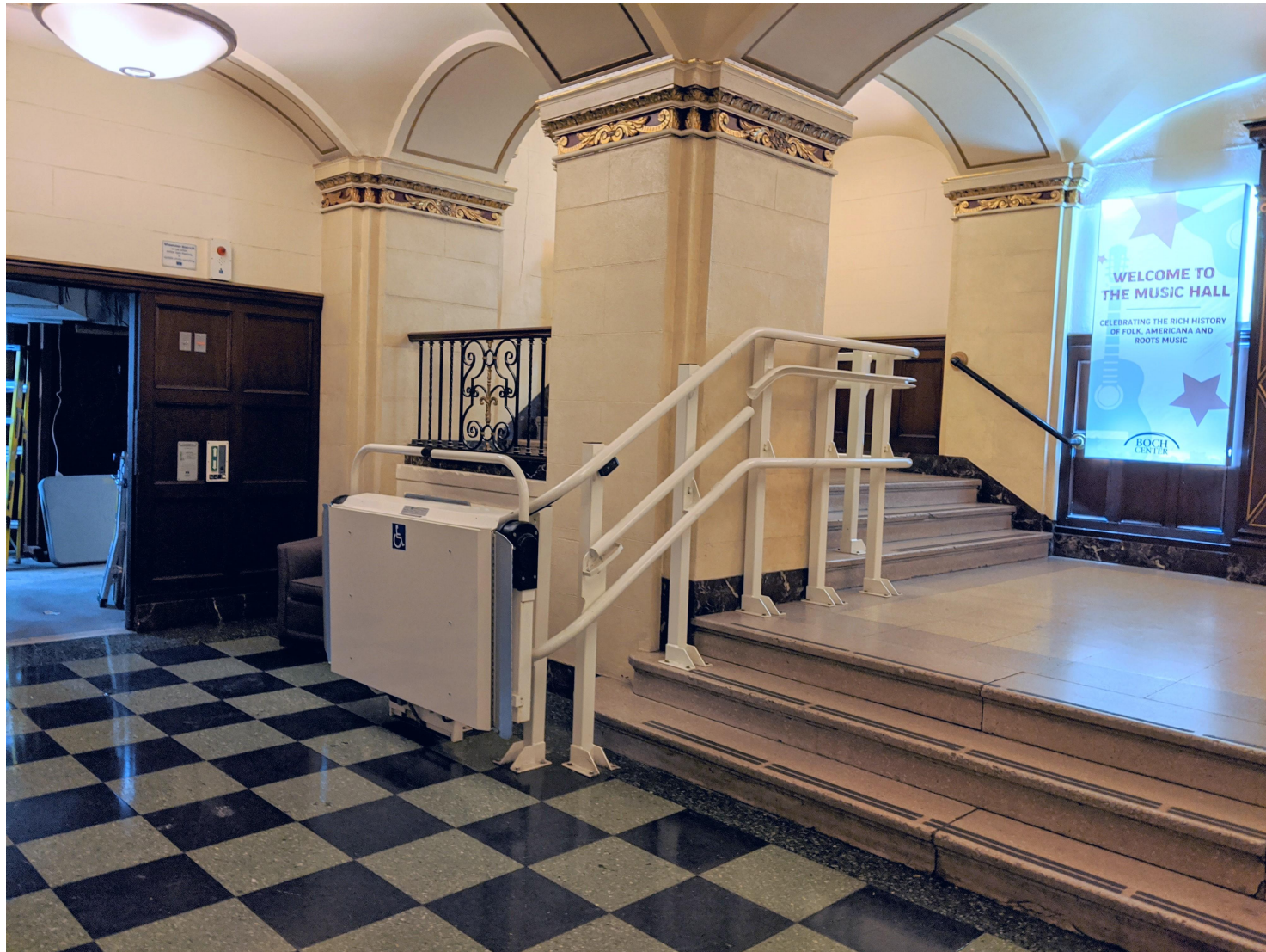
Portion of Stair Lift to Remain and Retrofitted to Access Intermediate Level
